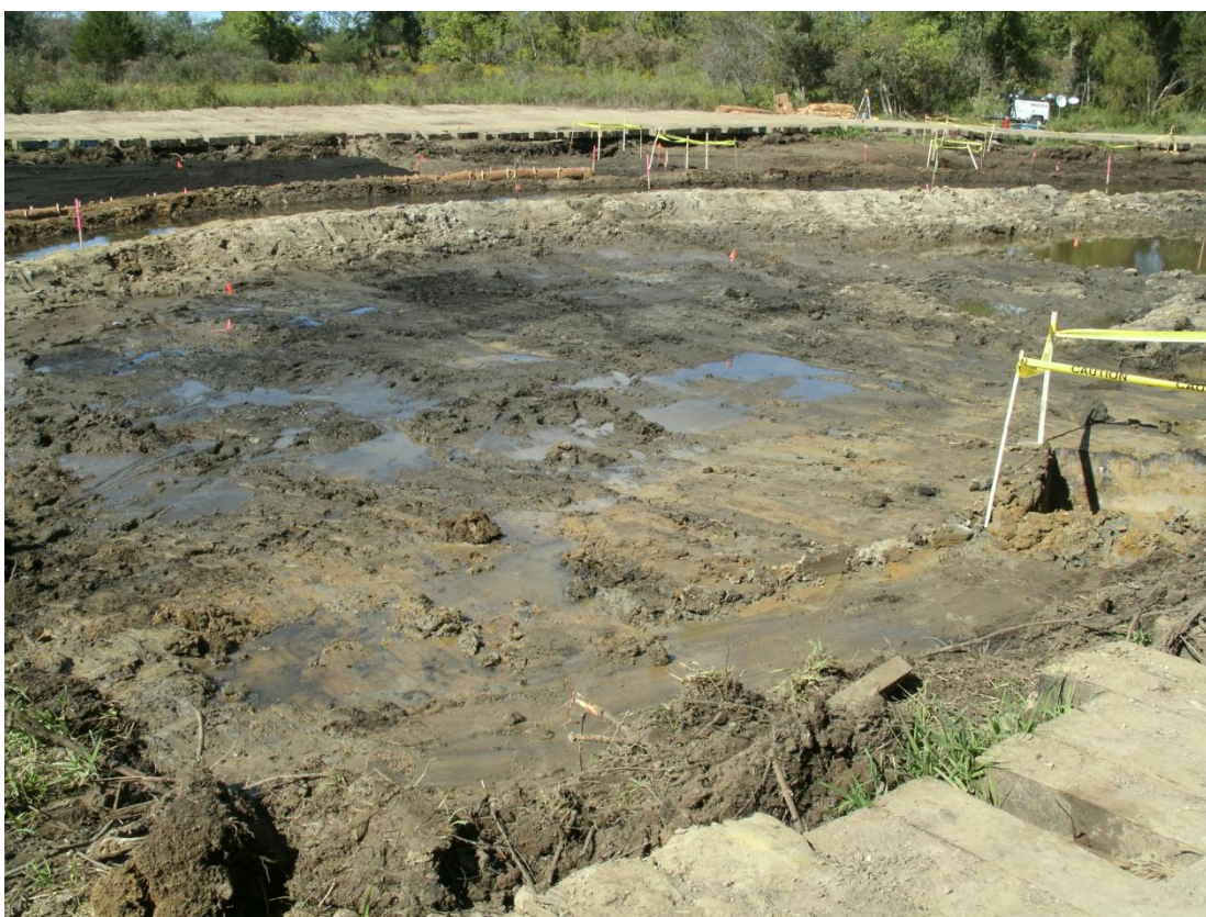
19+75R – 20+25R: Looking toward Talmadge Creek at area cleared for backfill (September 10, 2010)
