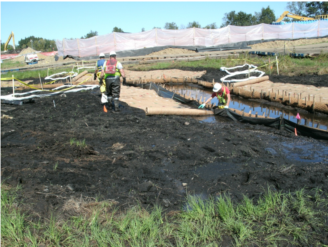
10+50L – 11+00L: Looking toward Talmadge Creek at seeding and mat placement (September 14, 2010)
