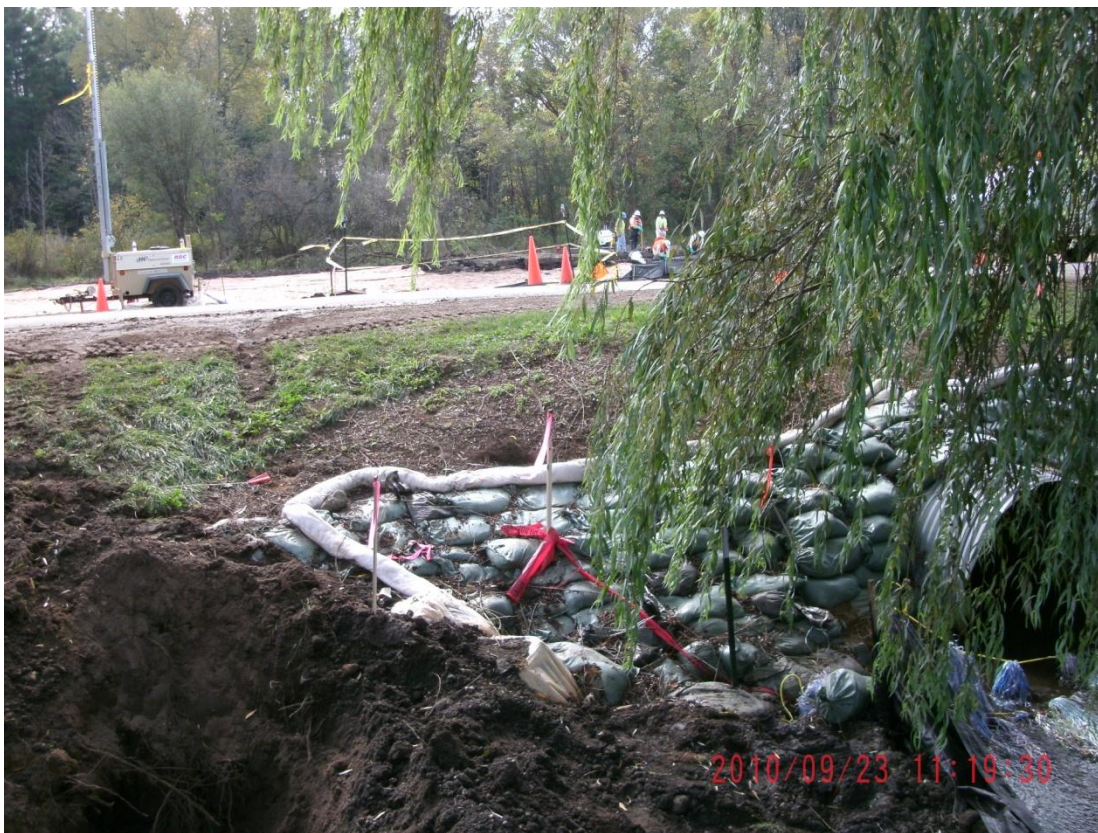
99+50R – 100+00R: Looking upstream with A Drive North visible in background (September 23, 2010)
