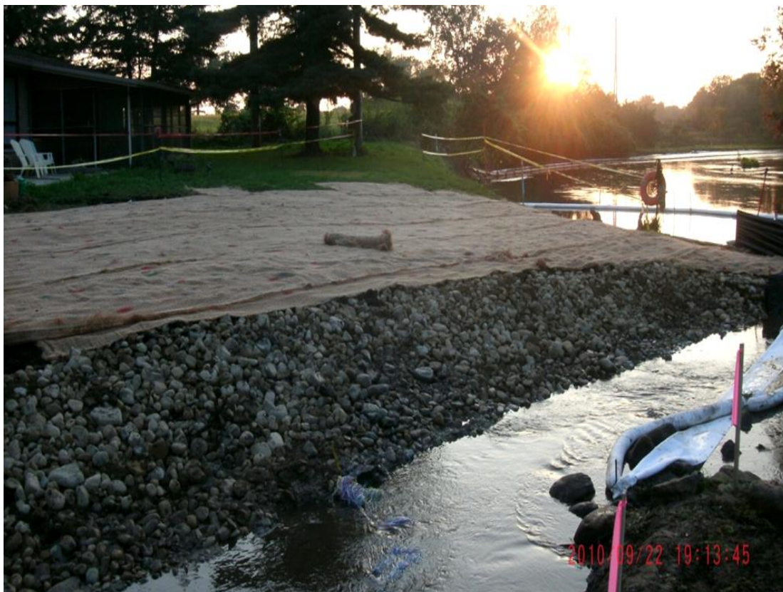
101+00R – 101+50R: Looking downstream across Talmadge Creek toward the Kalamazoo River (September 22, 2010)
