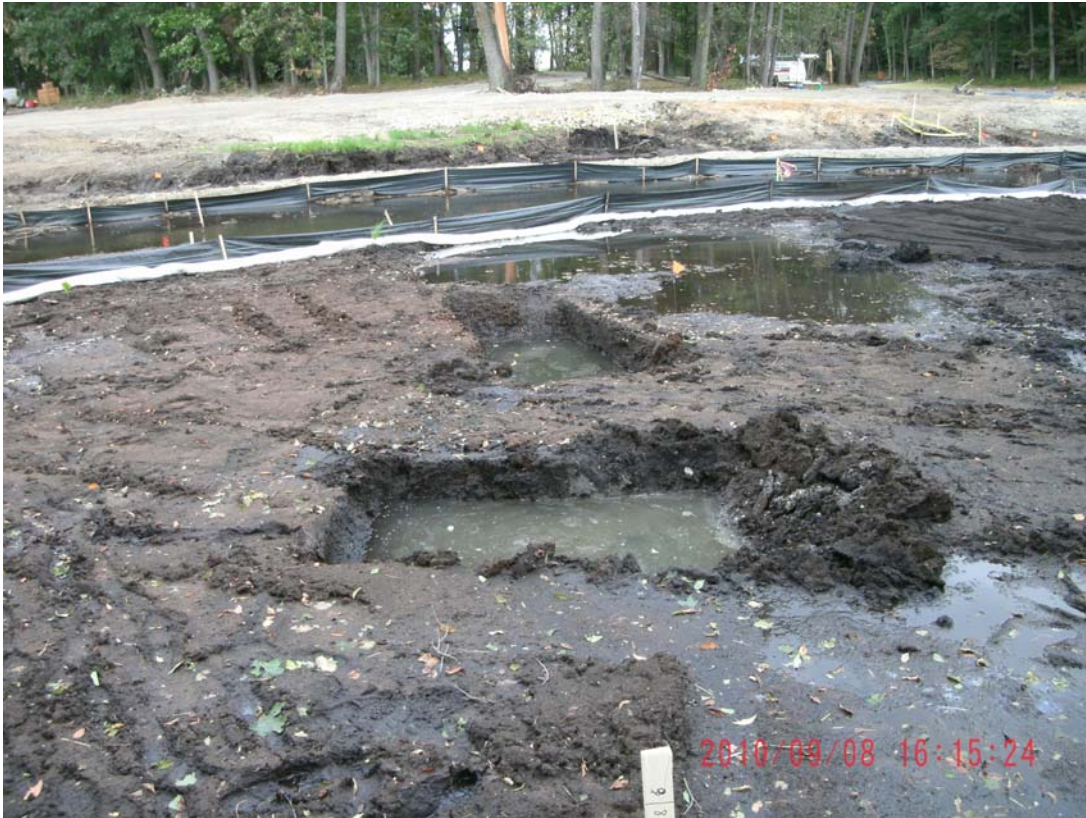
01+00L – 01+50L: Looking toward Talmadge Creek at 6-hour test pit prior to backfilling (September 8, 2010)
