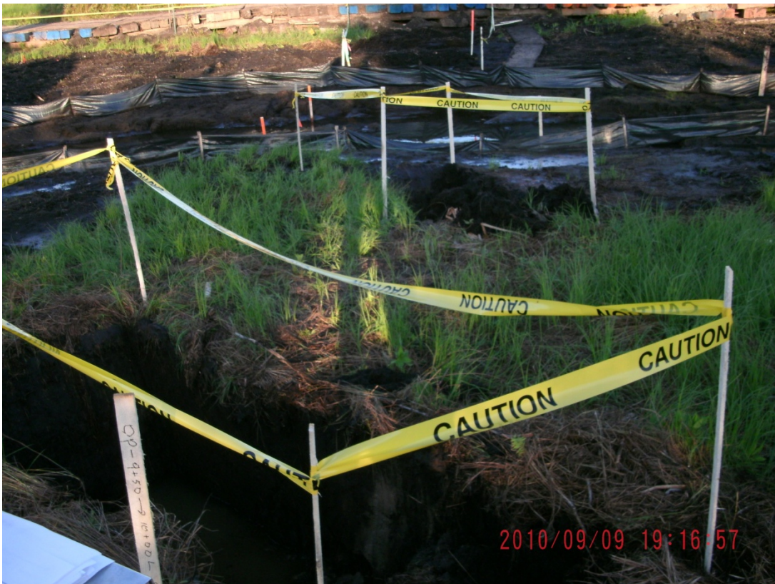
09+50L – 10+00L: Looking toward Talmadge Creek at 6-hour test and 48-hour observation pits (September 9, 2010)
