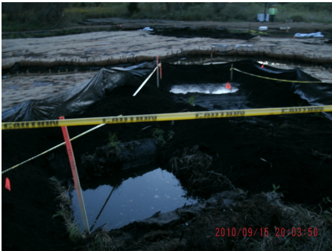
05+50R - 06+00R: Looking toward Talmadge Creek at 6-hour test and 48-hour observation pits prior to backfill (September 15, 2010)
