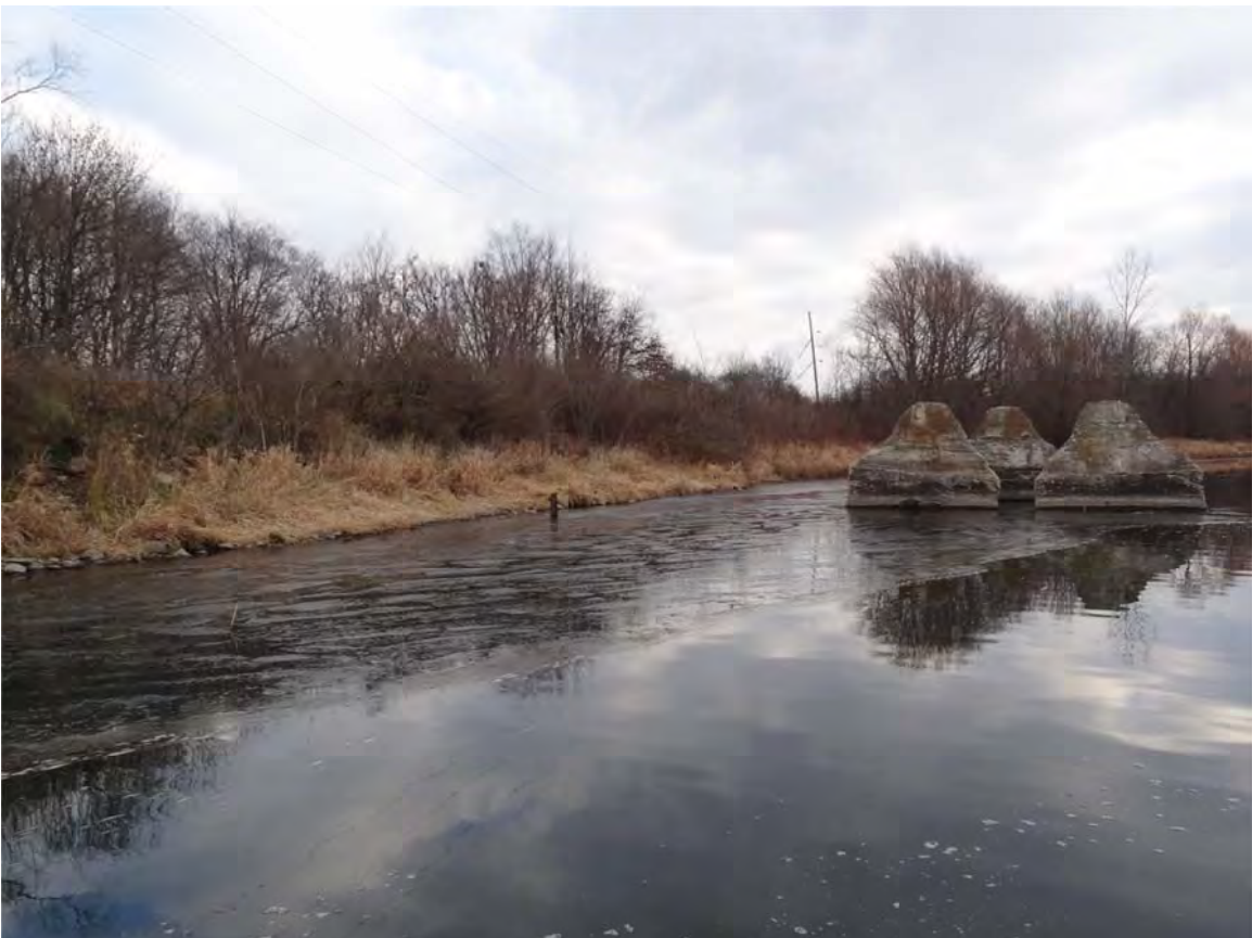
10. MP 5.63 RDB, ice observed along shoreline on upstream side of trestle.
