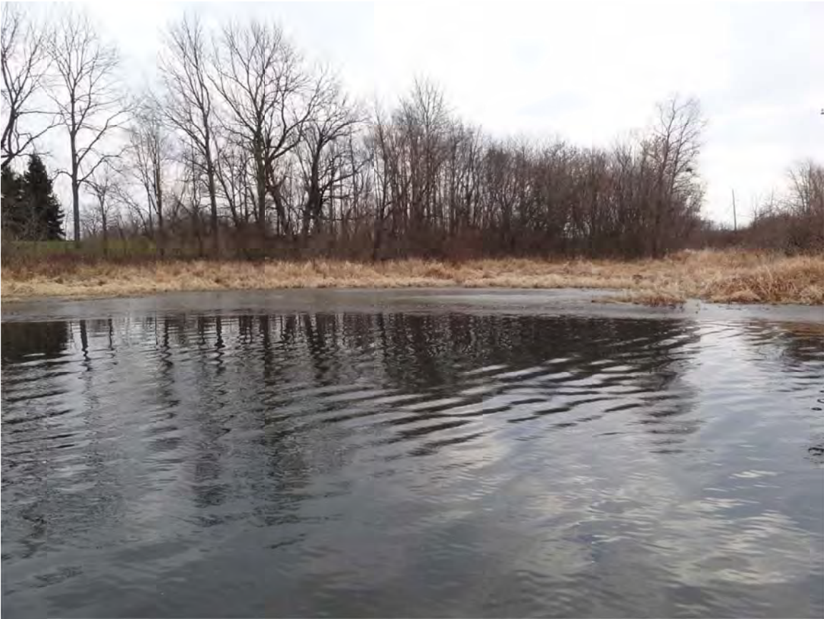
3. MP5.63 RDB, observed thin layer of ice on downstream side of trestle.
