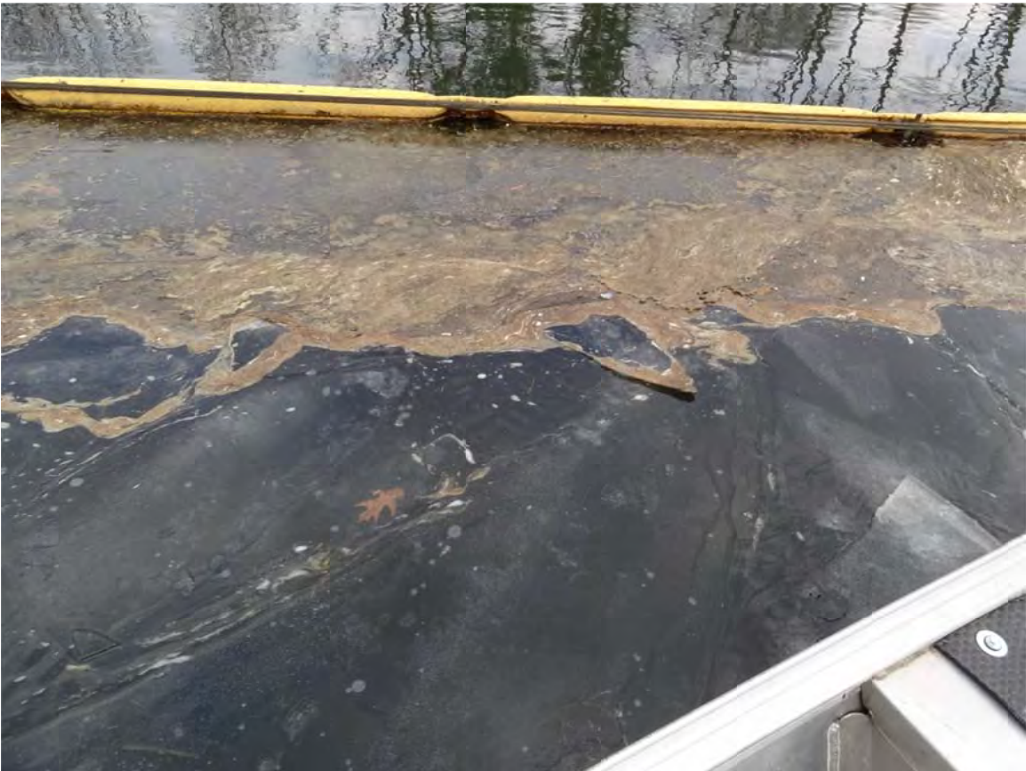
5. Ceresco Dam control point boom, some debris and ice observed.
