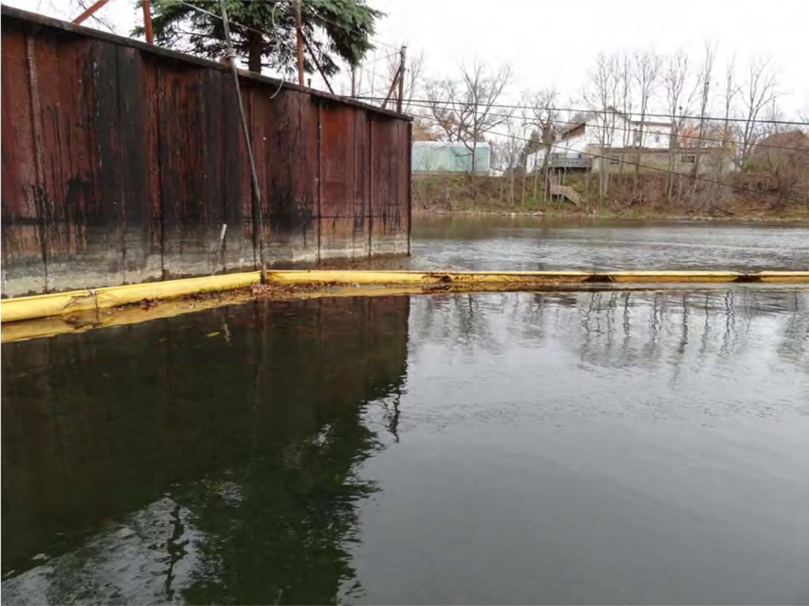
11. Ceresco Dam control point, sheen and tar globules observed.
