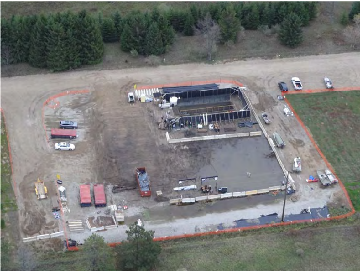
2. Frac-Tank City observed standing water.
