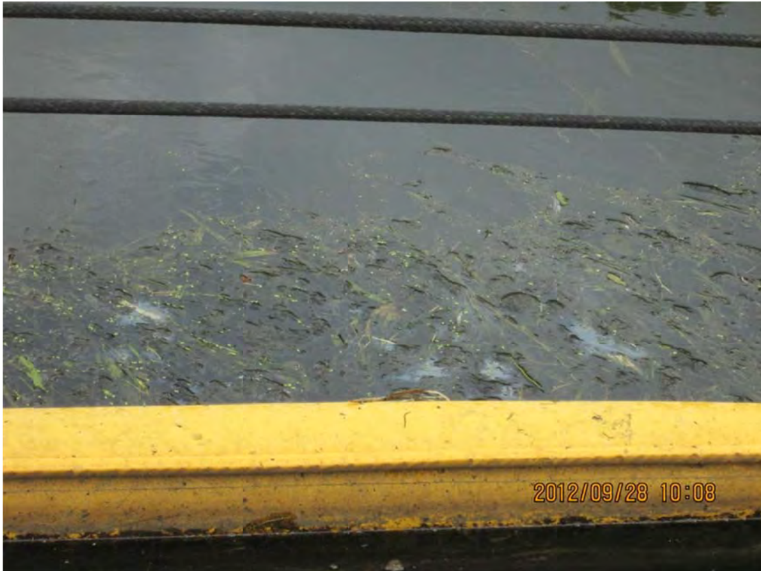
7. Sheen within debris in Ceresco Dam containment.
