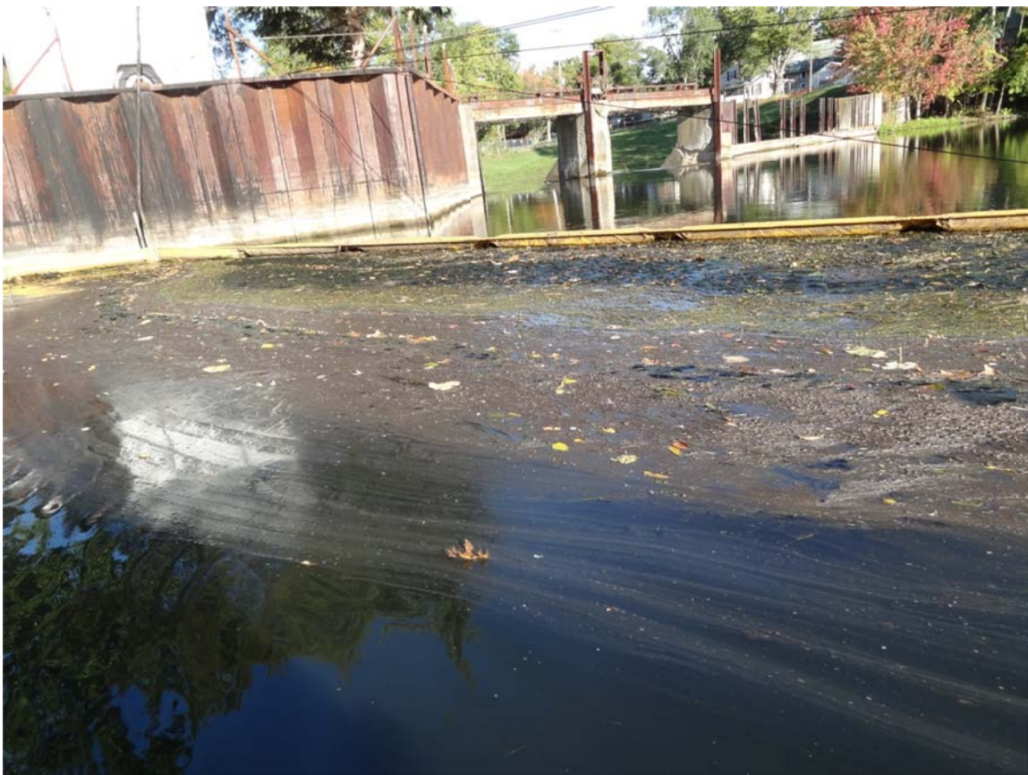
7. Ceresco Dam control point, debris and sheen observed within containment.
