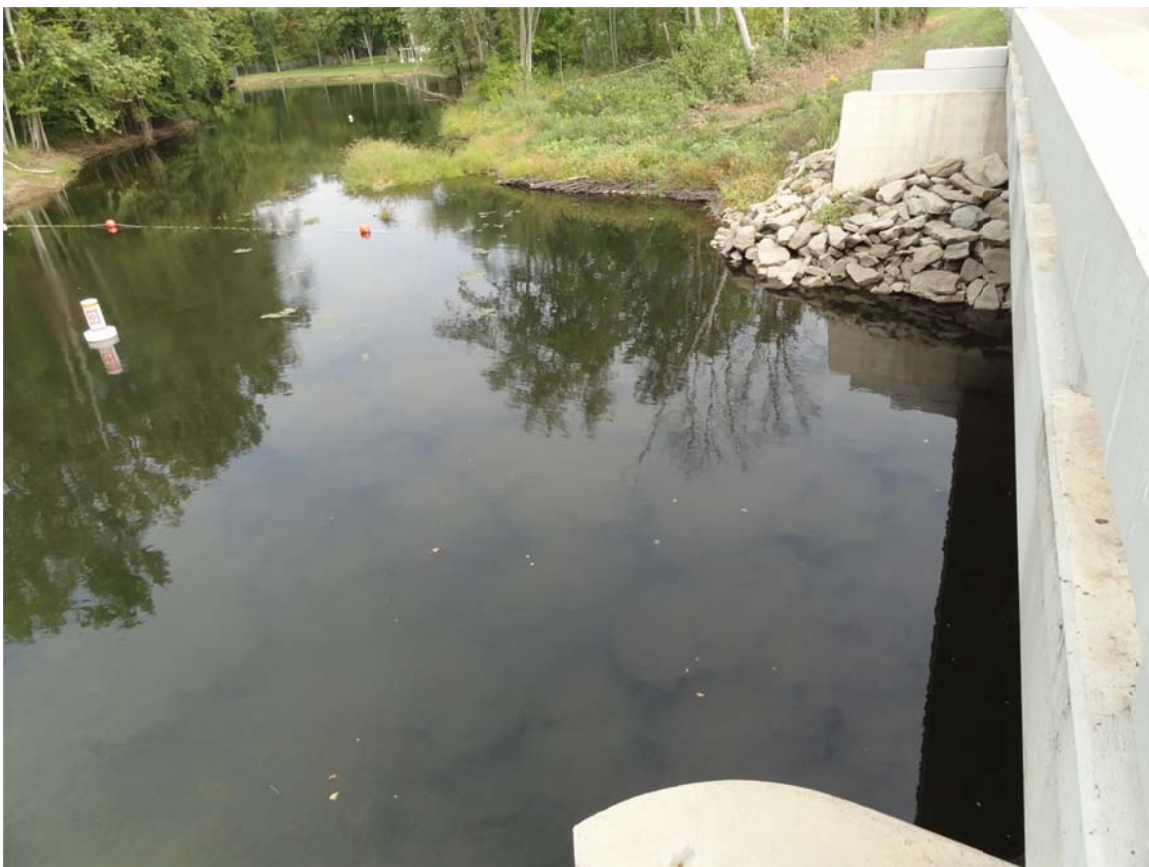
35. MP21.5 RDB Custer Drive Bridge sheen was observed.
