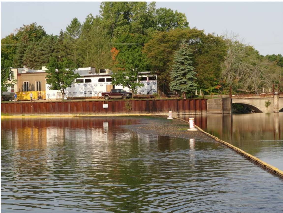
8. Observed debris collecting along control point boom at Ceresco Dam.
