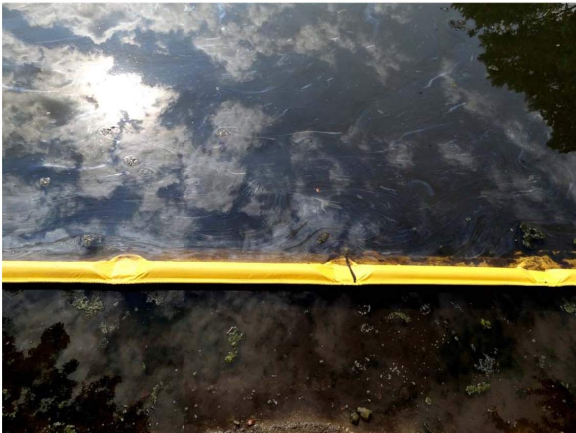
4. Sheen within containment along southern wall of Ceresco Dam.
