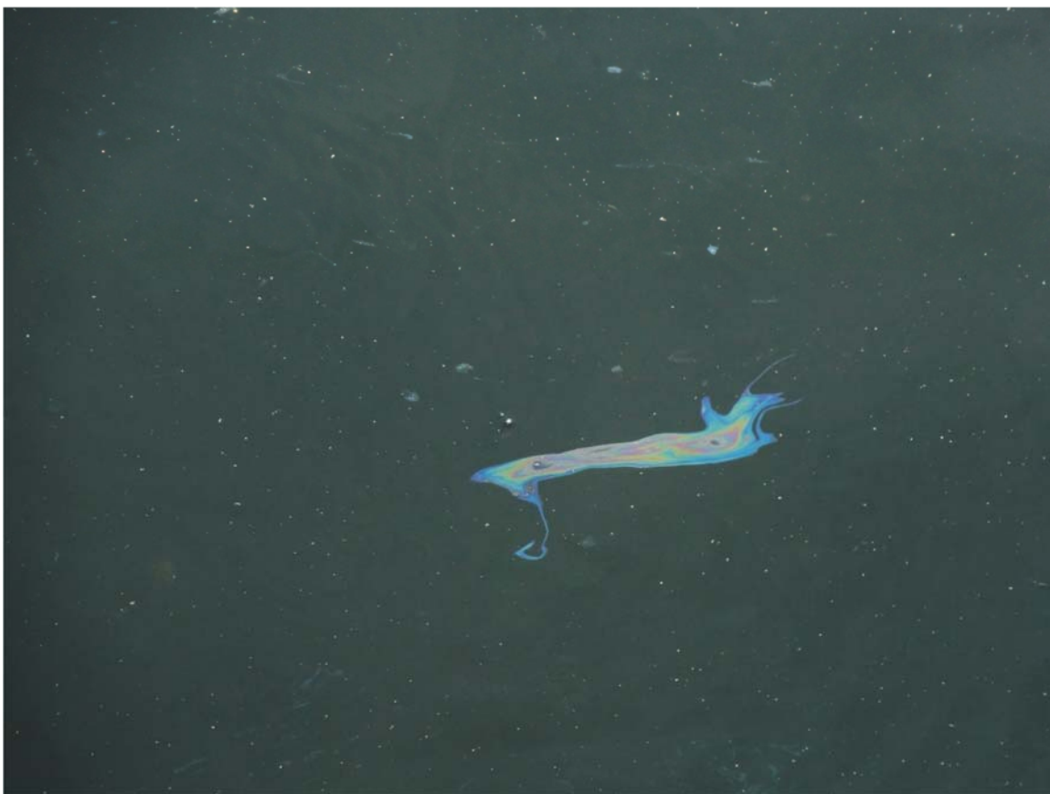
12. Ceresco Dam sheen observed.
