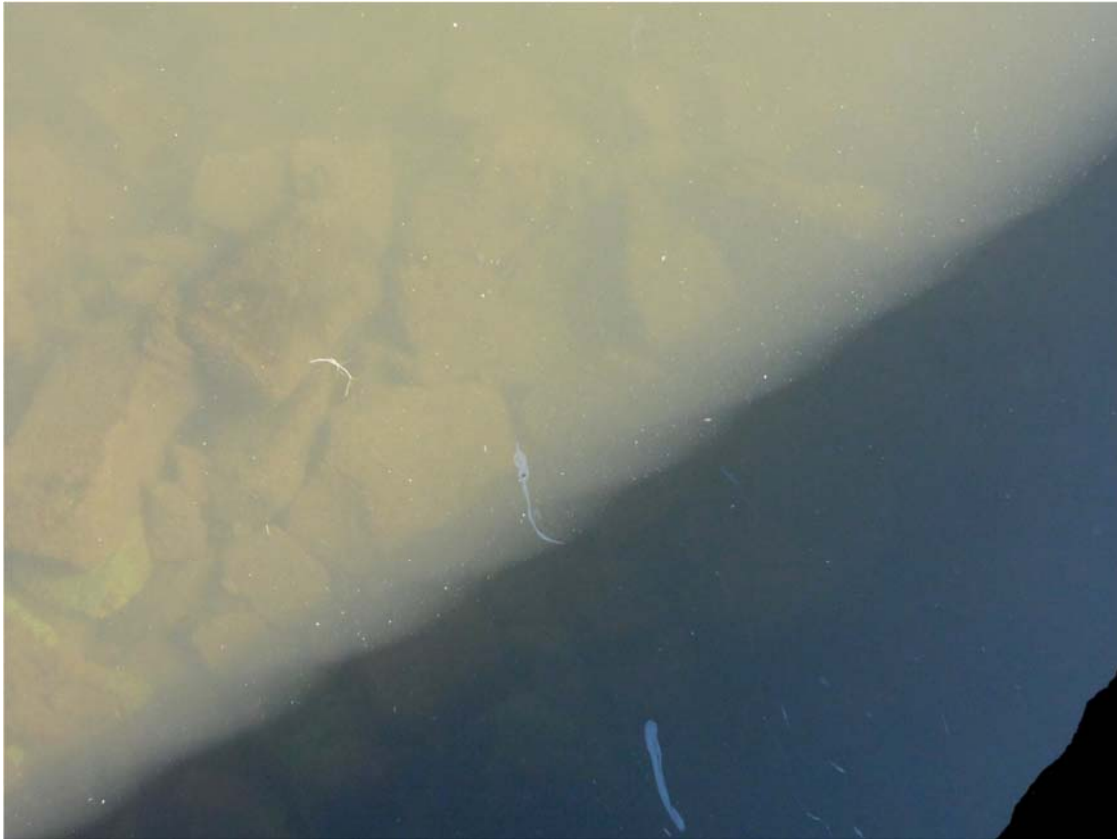
11. MP15.75 sheen observed flowing through culvert.
