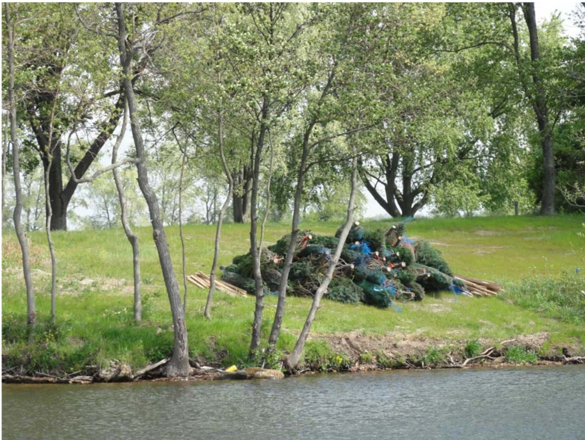
3. MP36.1 sediment control structure supplies staged near E4 boat launch.
