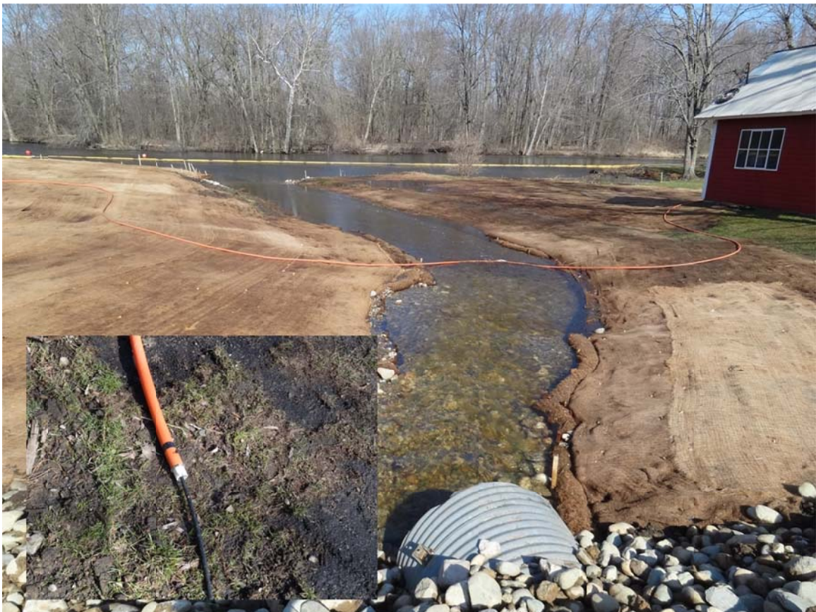
8. Talmadge Creek: coaxial cable running to house at Confluence.
