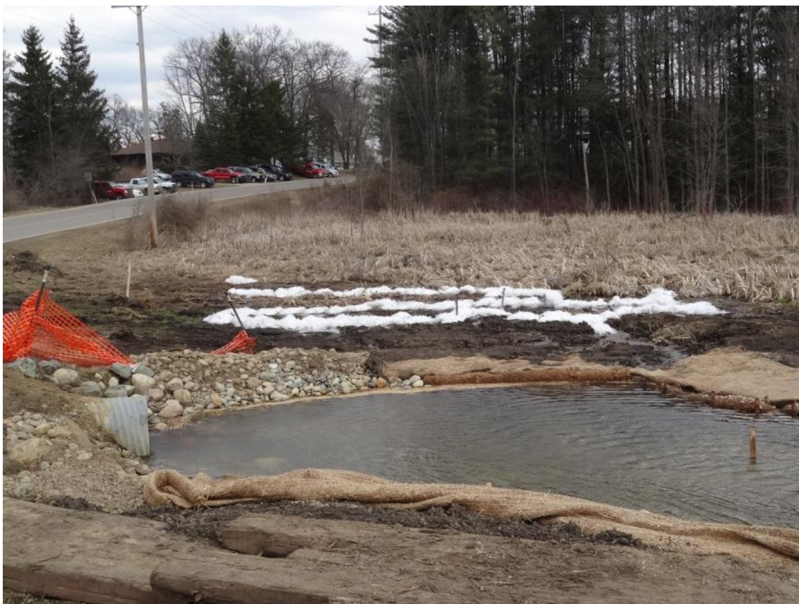
10. South of A Drive RDB overbank sheen observed.
