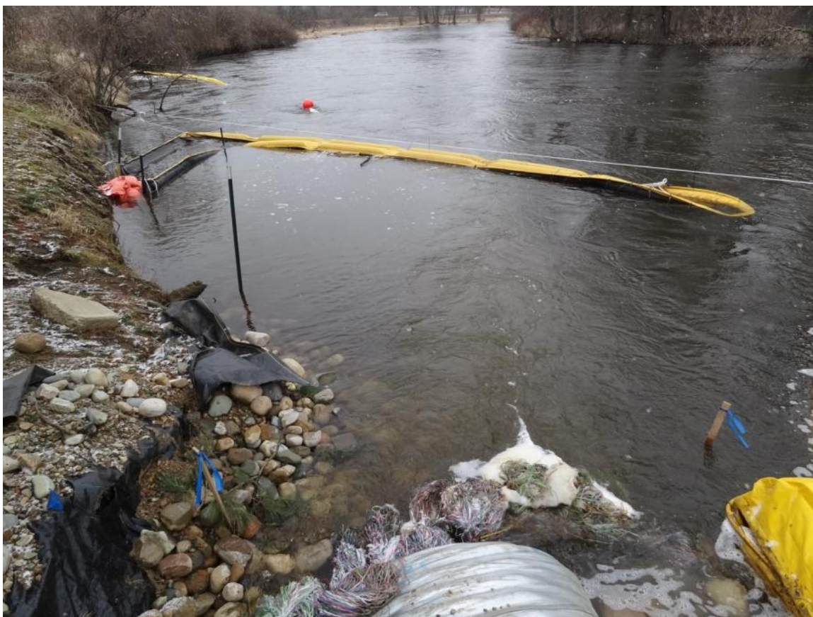
20. Confluence: bypass discharge.
