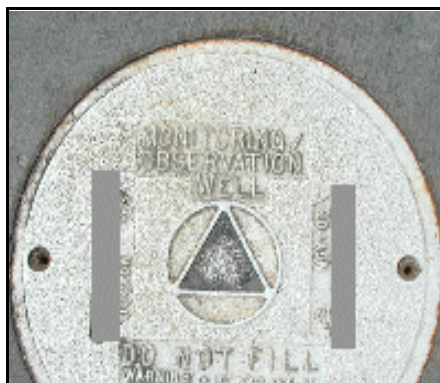
Sample Monitoring Well Cover
