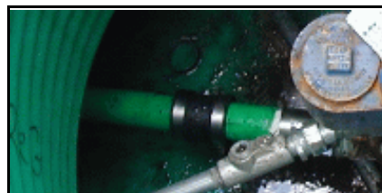
Closeup Of Flexible Piping In A Sump
