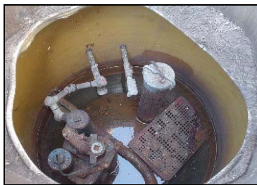
Contained sump with liquid and debris
