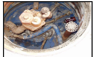
Flexible piping is kinked
