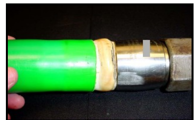
Flexible piping is bulging
