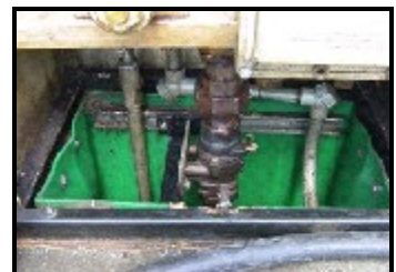
Contained dispenser sump
