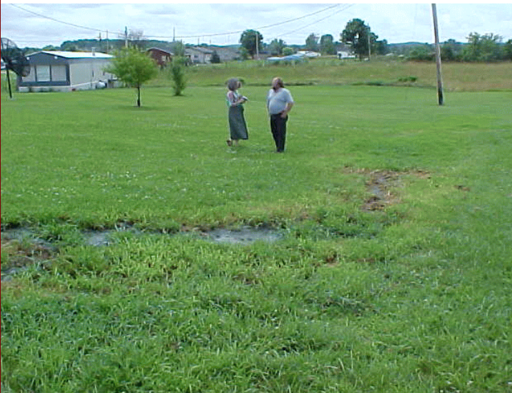
Failed Septic System: Preston, KY
