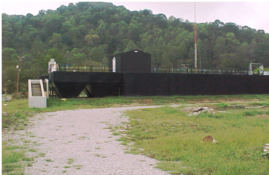
Figure 3: Package Plant, Hindman, Kentucky
