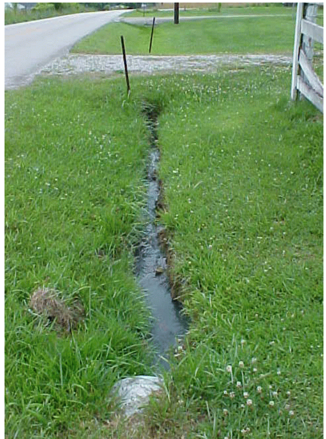
Straight Pipe Drainage: Preston, KY
