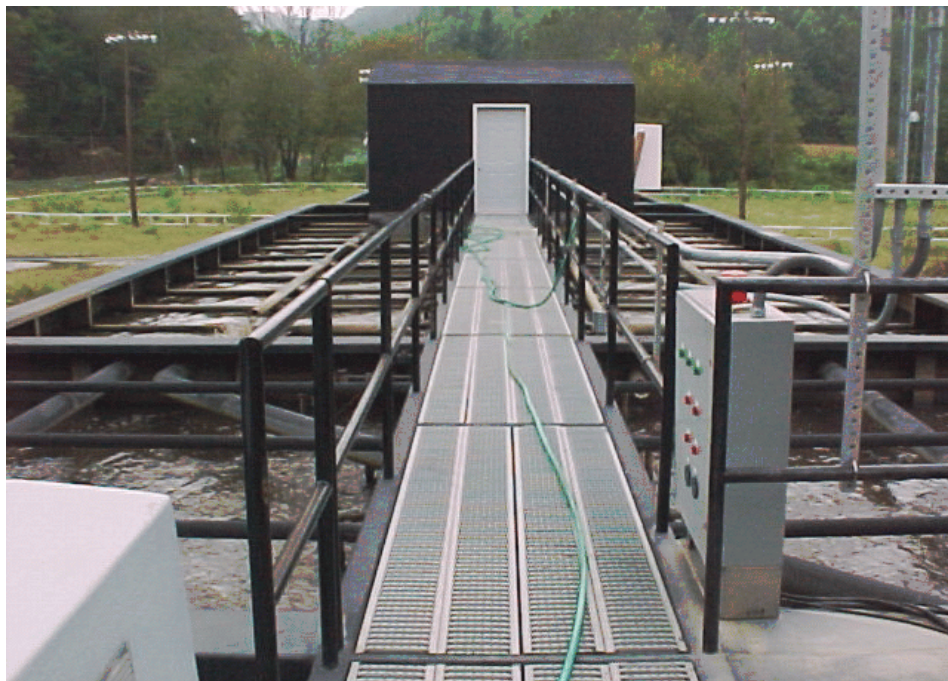
Figure 4: Aeration Tank, Hindman, Kentucky
