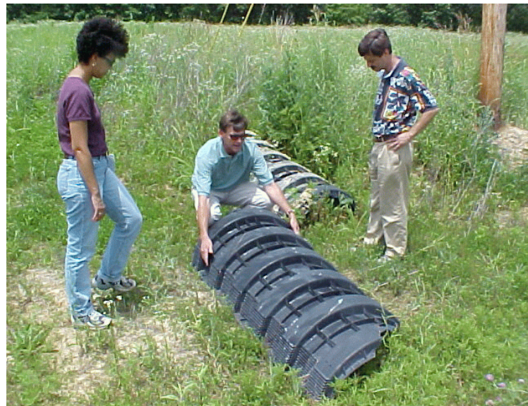
Infiltrator Drainage System: Preston, KY
