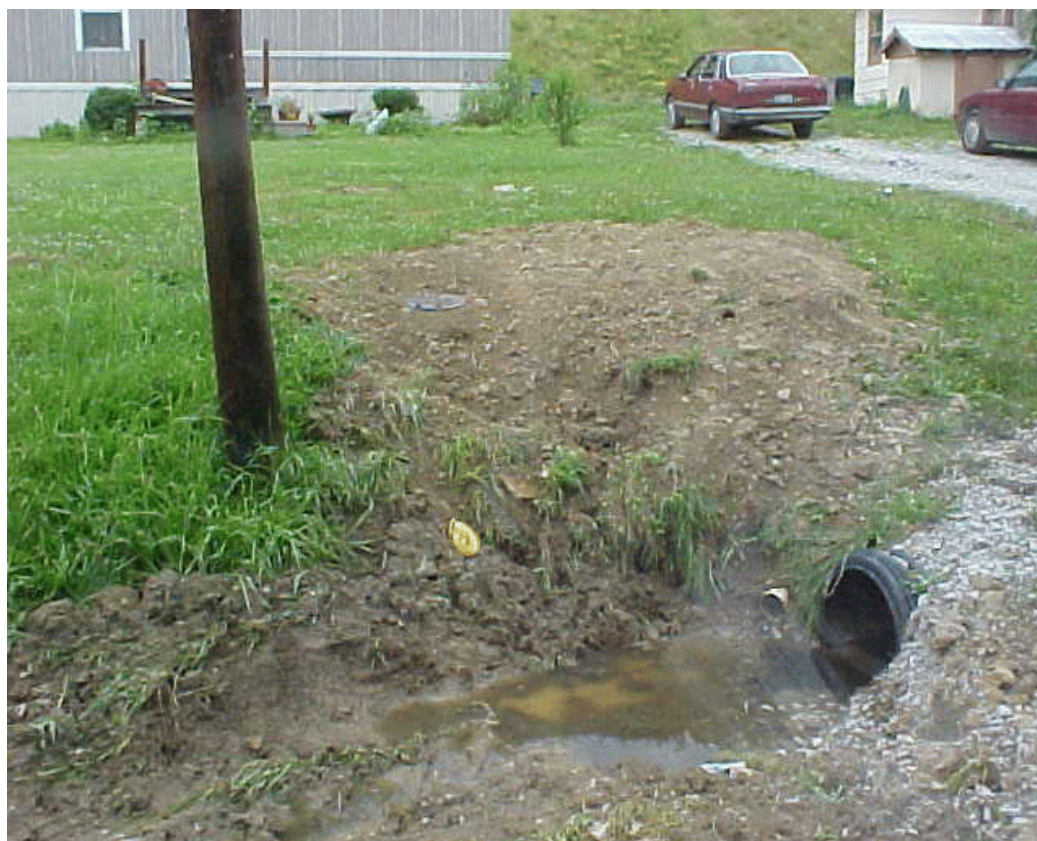
Straight Pipe:Martin County, KY
