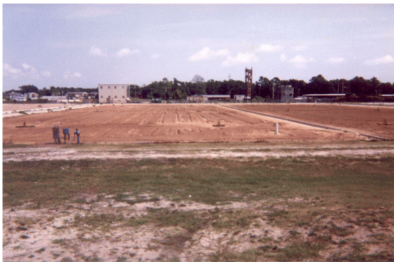
Intermittent Sand Filters
