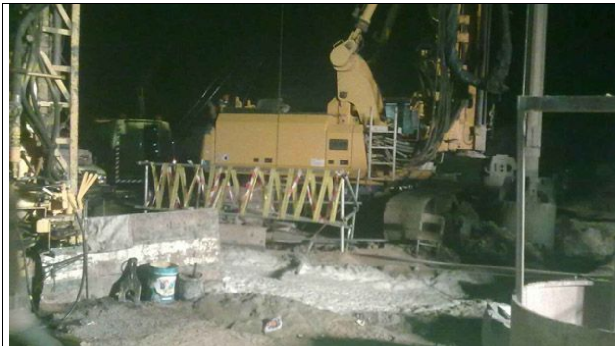
The company digging close to the Taif bore well in which a woman has been trapped is preparing to dig an artesian well to reach the woman's body. (AN photo)
