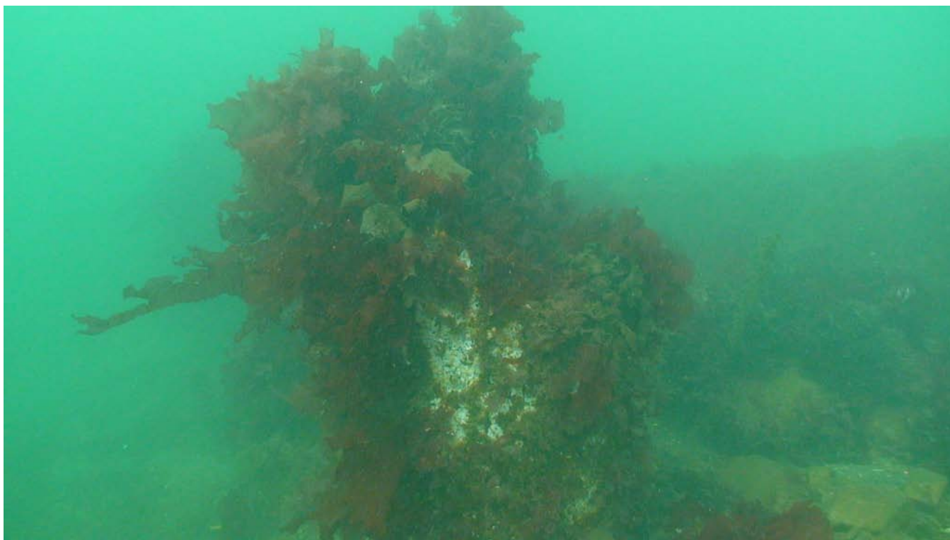
Close up view of a piling, broken off near the bottom.
