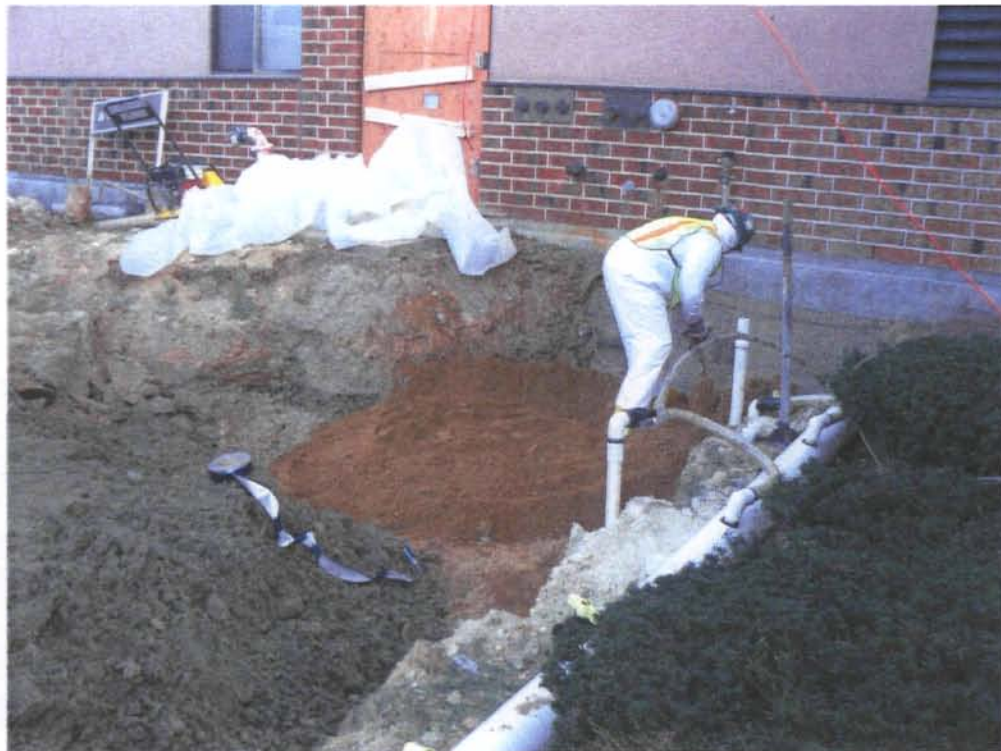
Description: Building connection Name: 15Dec2010 004
