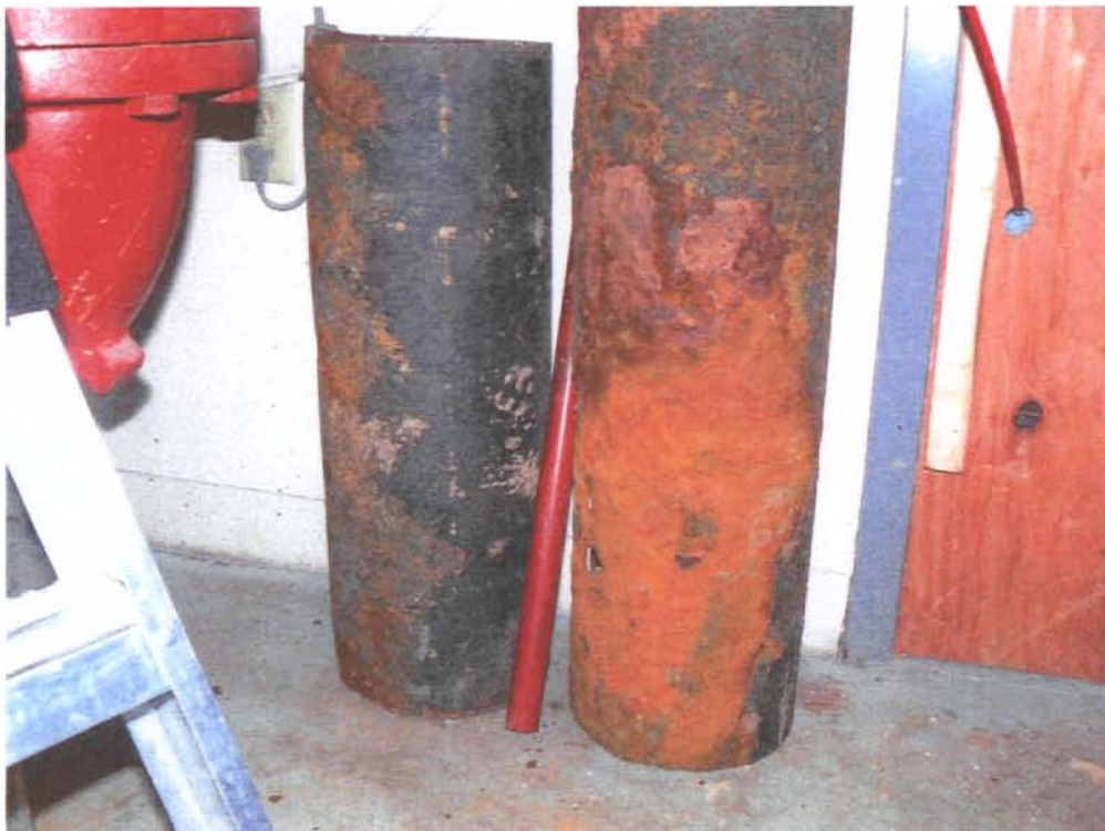
Description: Section of corroded waterline Name:
