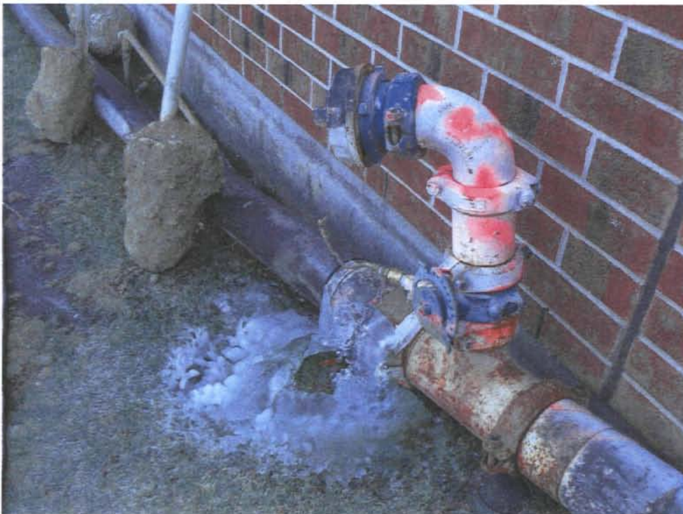
Description: Temporary waterline icing Name: 17Dec2010 004
