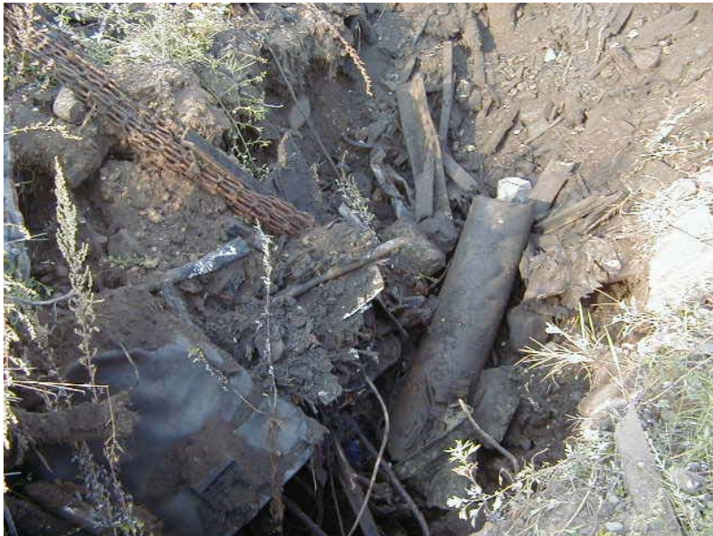
Photo No. 6C: Debris In Excavation
