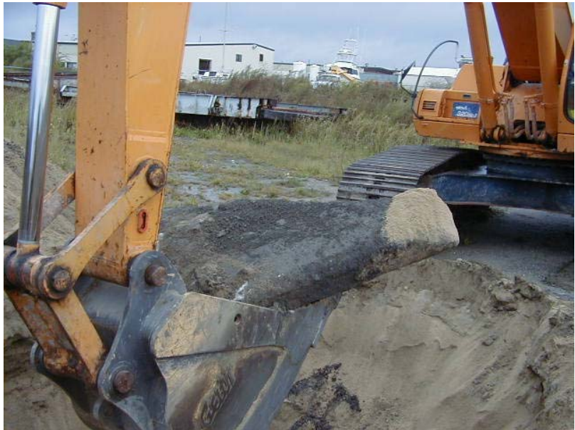
Photo No. 7A: Large Piece of Concrete Debris (TP-D7)
