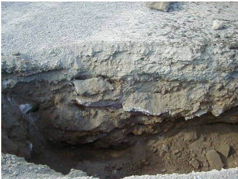
Photo No. 7F: Concrete Debris Near Ground Surface (TP-D10)
