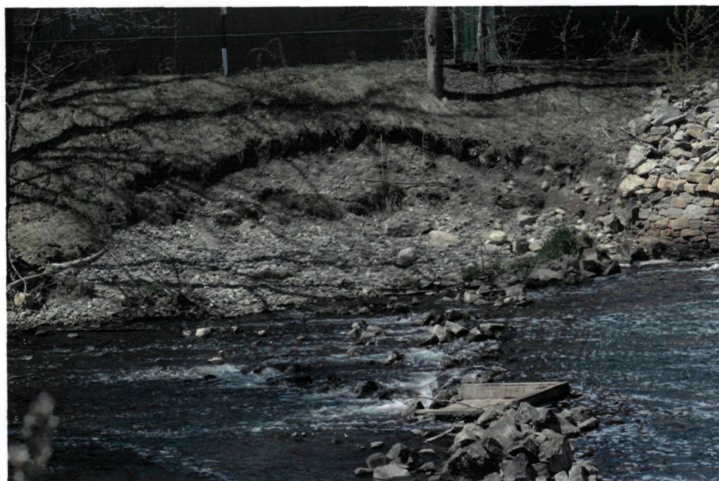
Figure 6. Scarp immediately below Allendale Dam on the west side of the Woonasquatucket River, April 18, 2006.
