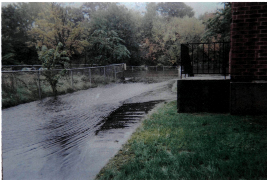
Figure 9. Service drive on south side of Centredale Manor on October 15, 1005. The elevation of the flooded area of the driveway is approximately 97.5 ft according to the as-built plans.
