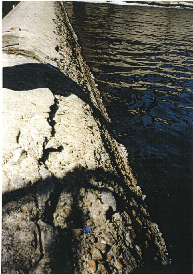
Photo 5: Severe and extensive spalling, measuring up to 8" deep, on the downstream face for the entire length of the spillway.
