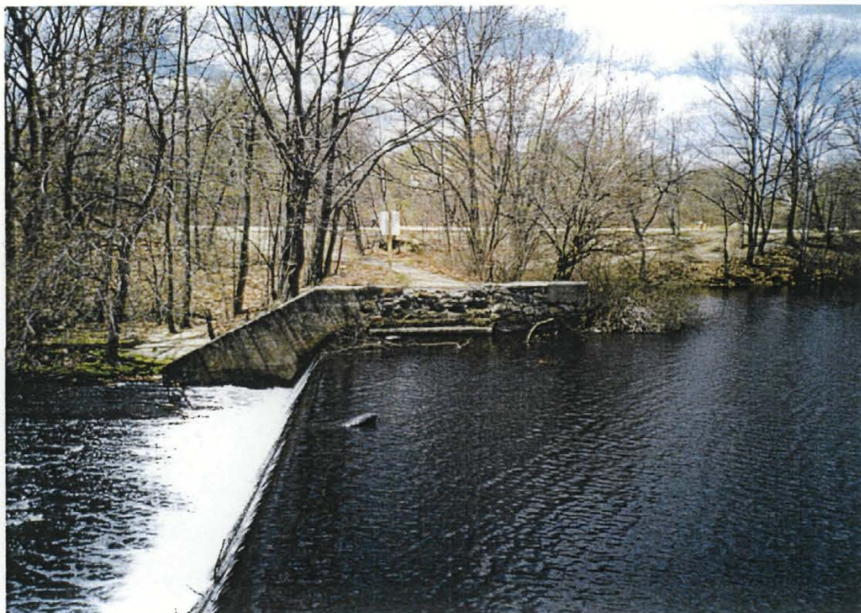
Photo 1: Concrete facing of the stone core wall has spalled off at the west abutment wall. Note: the debris caught at the 12x12 timber beam of the old spillway wall.
