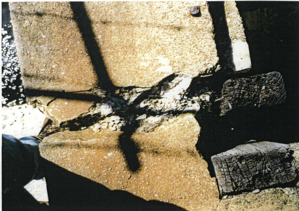
Photo 2: Severe concrete deterioration of the concrete at the timber gate guides of the left outlet structure.
