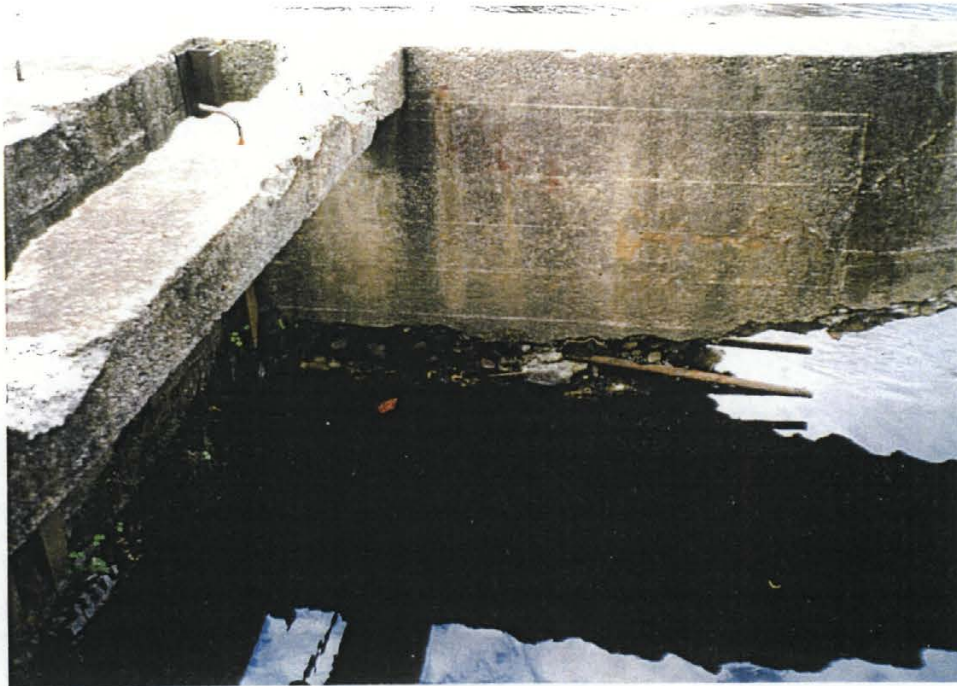
Photo 3: 6' long x 3' high x 1'-4" deep spill with exposed rebar at the east abutment wall. Note: the deteriorated concrete around the gate stem opening of the gate structure.
