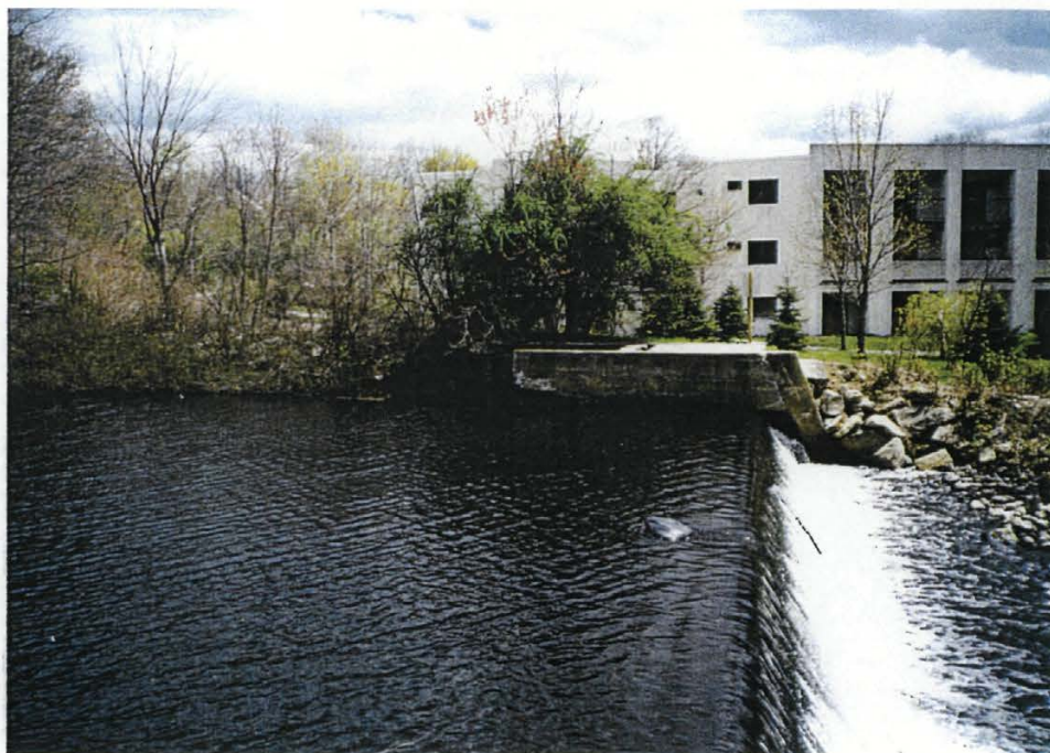
Photo 2: East abutment wall. Note: the spall with exposed rebar at the upstream/leading end of the wall.
