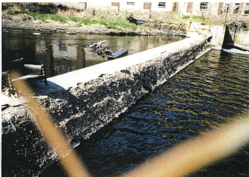
Photo 4: Downstream view of the spillway. Note: the debris upstream of the spillway.
