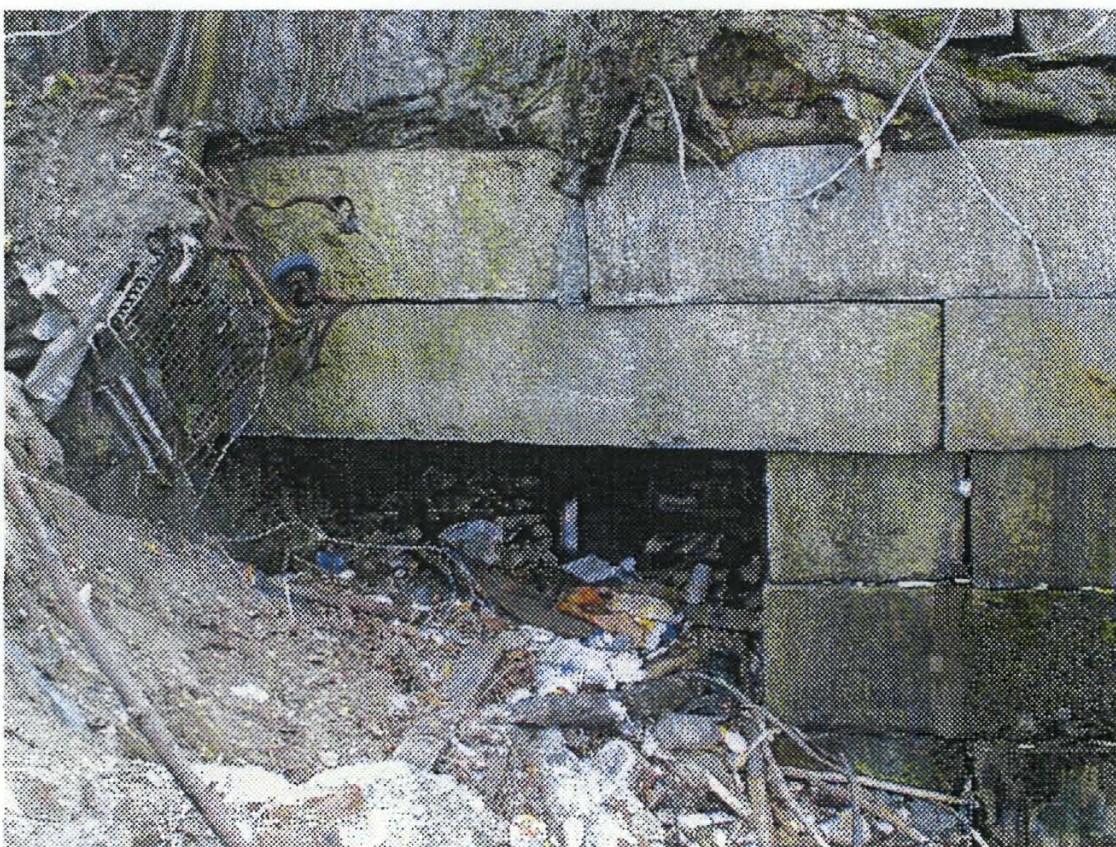
Photo 4 – Outlet works are filled with debris and earth.
