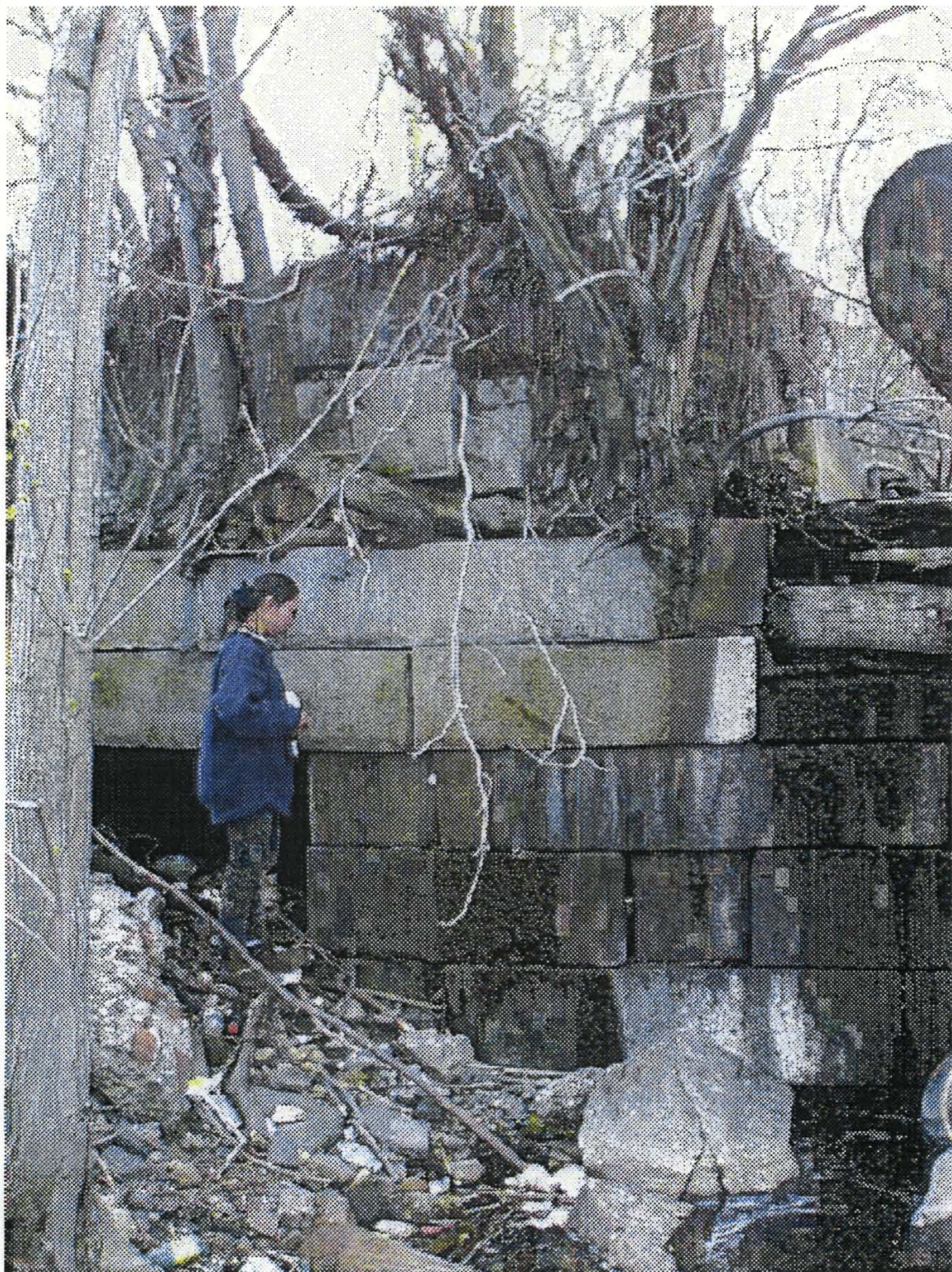
Photo 5 – Shifted blocks on right embankment and downstream side of outlet works.
