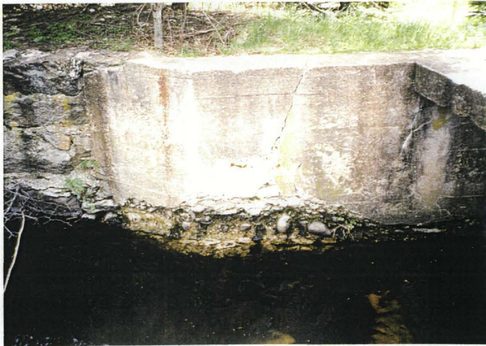
Photo 4: Two full height cracks, measuring up to 1/2" thick x 1'-4" deep at the east training wall of the gate structure. Note: the deteriorated concrete, up to 3" deep, at the bottom of one of the cracks.
