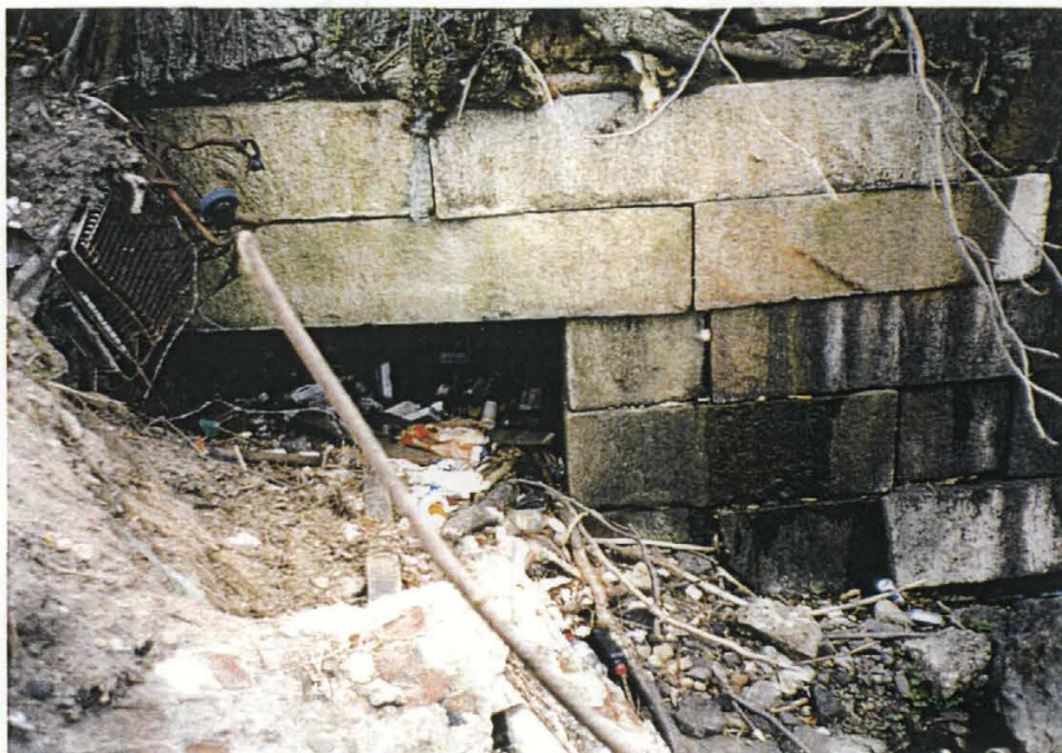
Photo 1: Debris almost completely fills the opening of the outlet structure located at the right side of the spillway.
