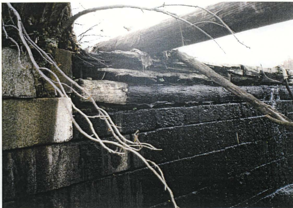
Photo 3: Severely weathered and cracked 10x10 timber at the top of the spillway adjacent to the outlet structure.
