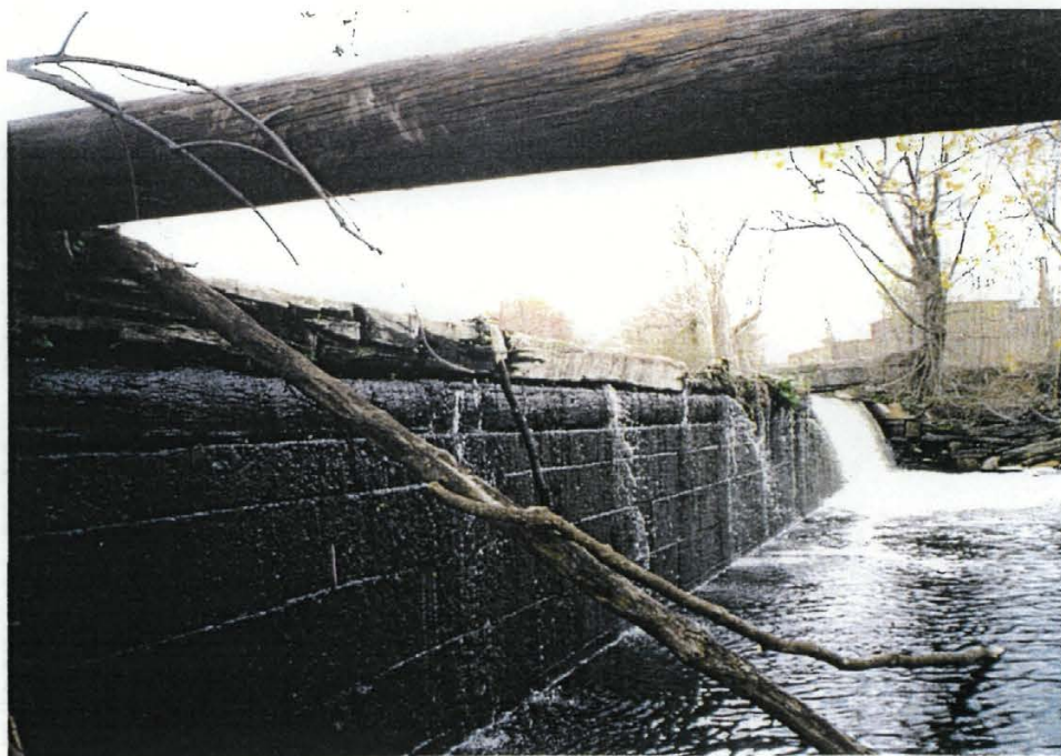
Photo 4: A large telephone pole and other minor tree debris caught at the top of the spillway. Note: seepage through the gaps between the 10x10 and the tree trunk.
