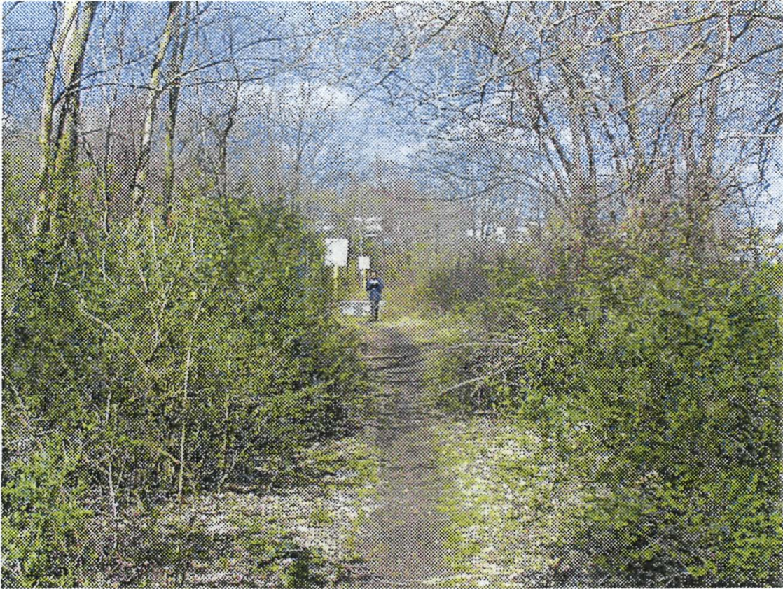
Photo 3 – Dam crest on left embankment showing heavy tree and brush growth.
