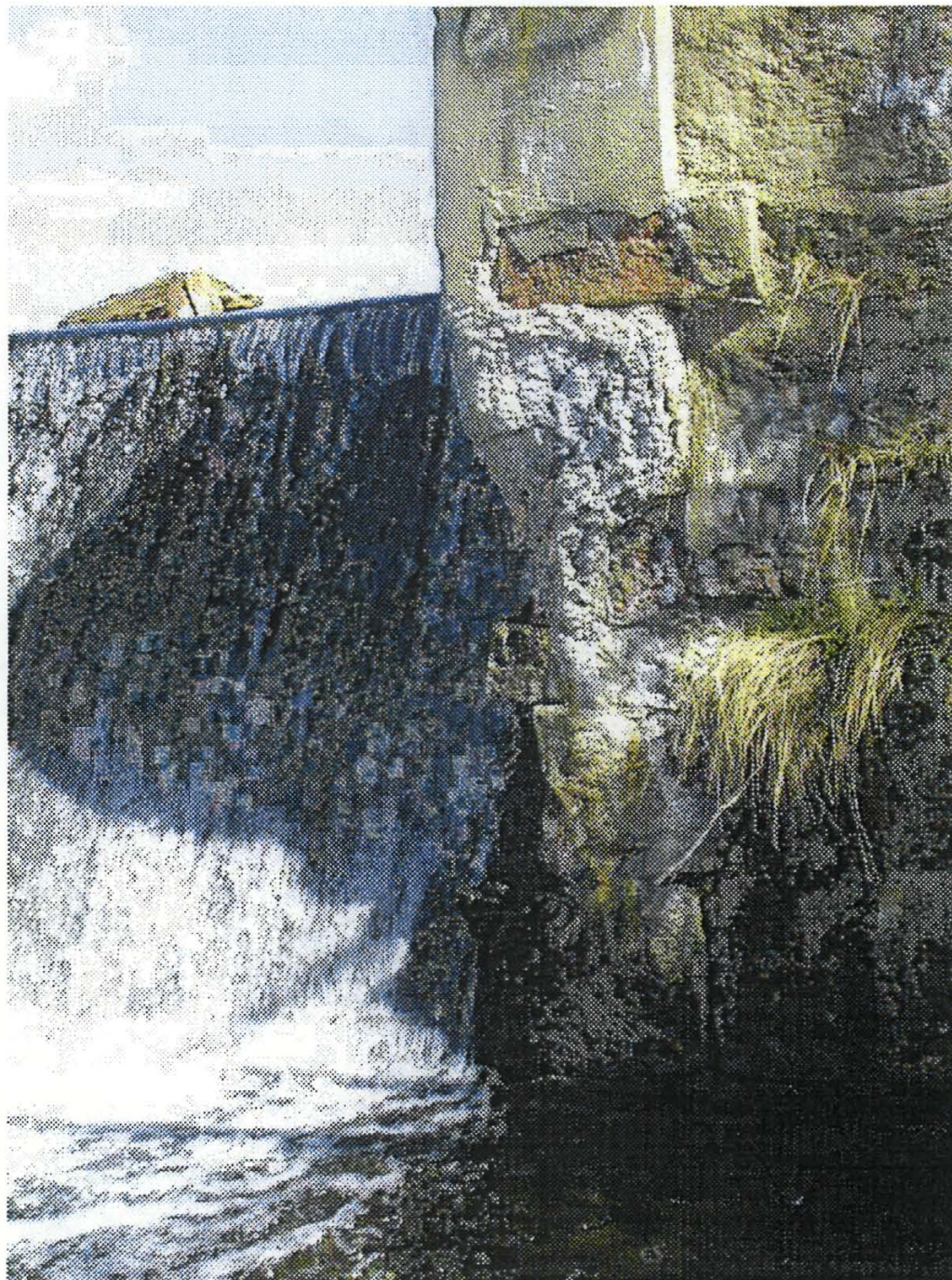
Photo 7 - Spalling concrete on outlet works on left side of spillway.
