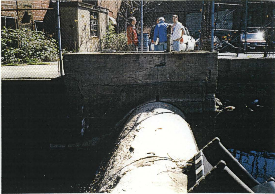
Photo 1: Numerous hairline cracks with efflorescence on the left wall of the outlet structure.
