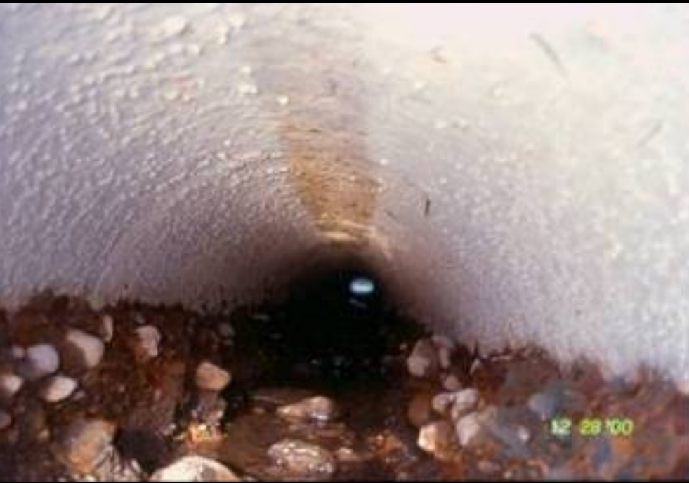
24" Round Culvert (inadequate flow)
