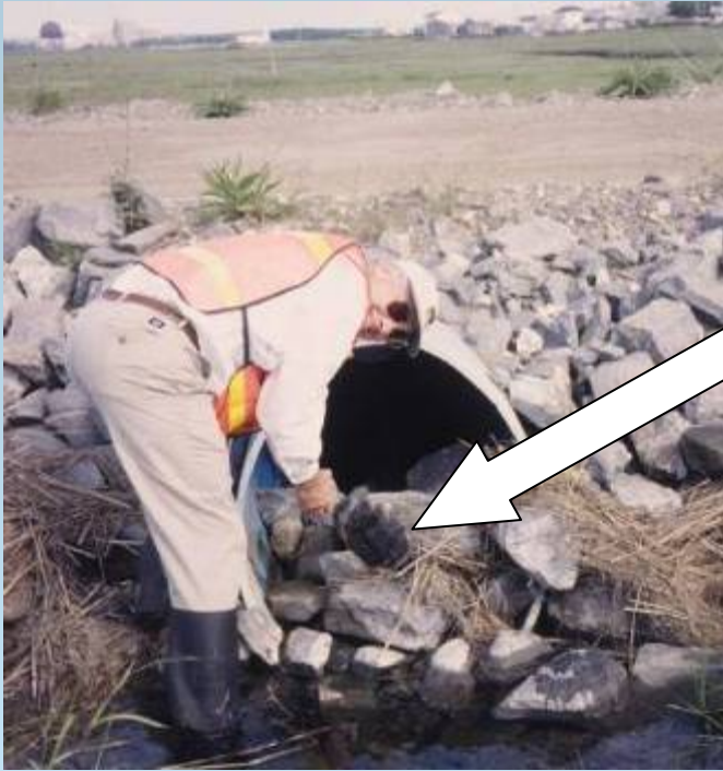
Rocks Block Pipe
