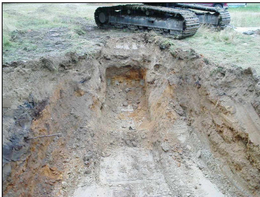
Photograph 12 RRA of contaminated soil at Area A
