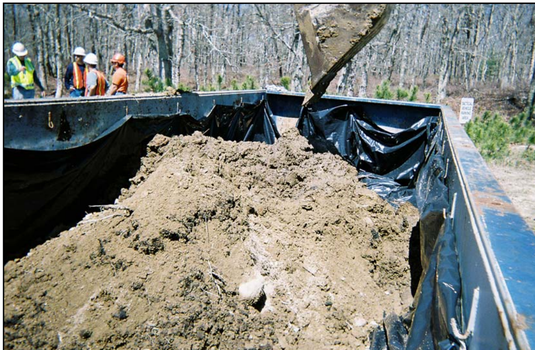
Photograph 15 Contaminated soil from RRA at Area E
