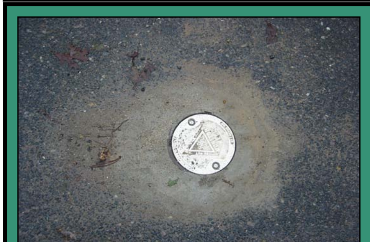
A flush-mounted monitoring well
