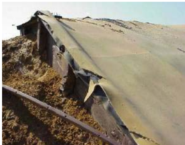
Figure 5-4. Example of Damage to STAPP™ Support Frame (photo not taken at Camp Edwards)
