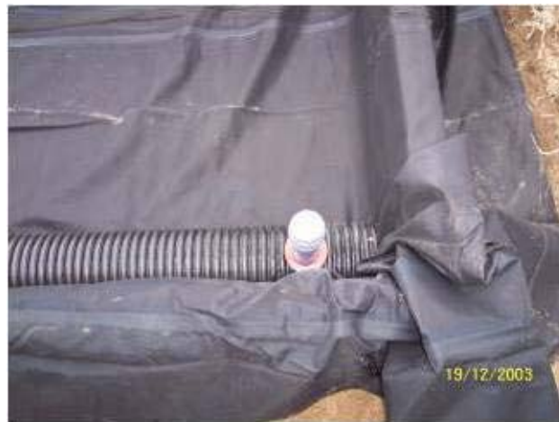
Figure 4-4. Internal Water Reservoir System
