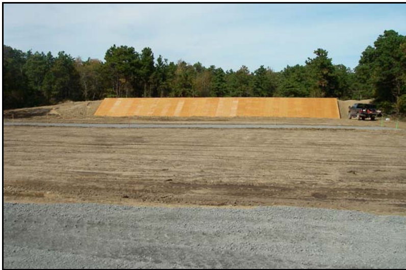
Figure 3-2. Juliet Range Installed with STAPP™
