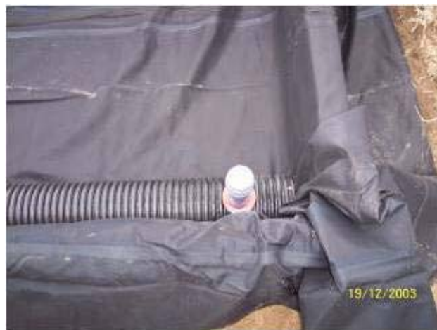
Figure 5-3. Internal Water Reservoir System
