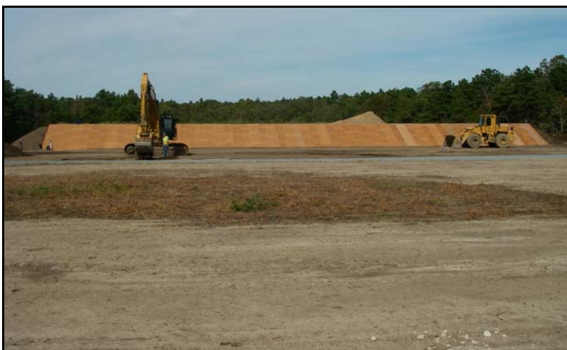
Figure 3-3 Kilo Range Installed with STAPP™
