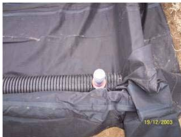
Figure 4-4. Internal Water Reservoir System
