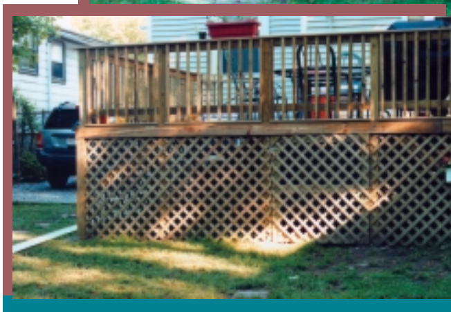
Top: Before—bare soil under porch deck. Bottom: After—area barricaded with lattice and trim.
