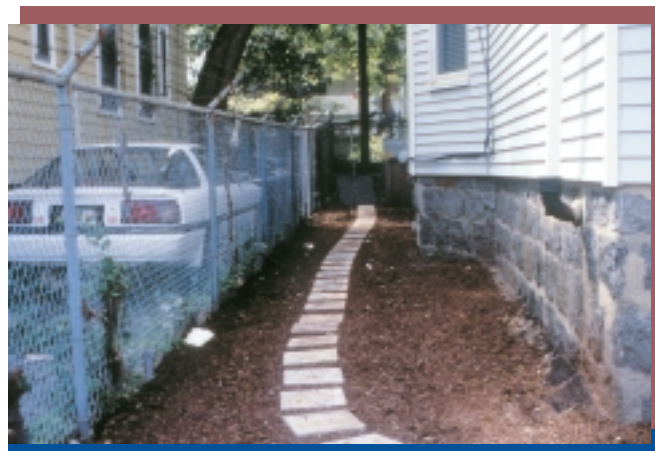
Install stepping stones to prevent contaminated soil from being tracked into the house.
