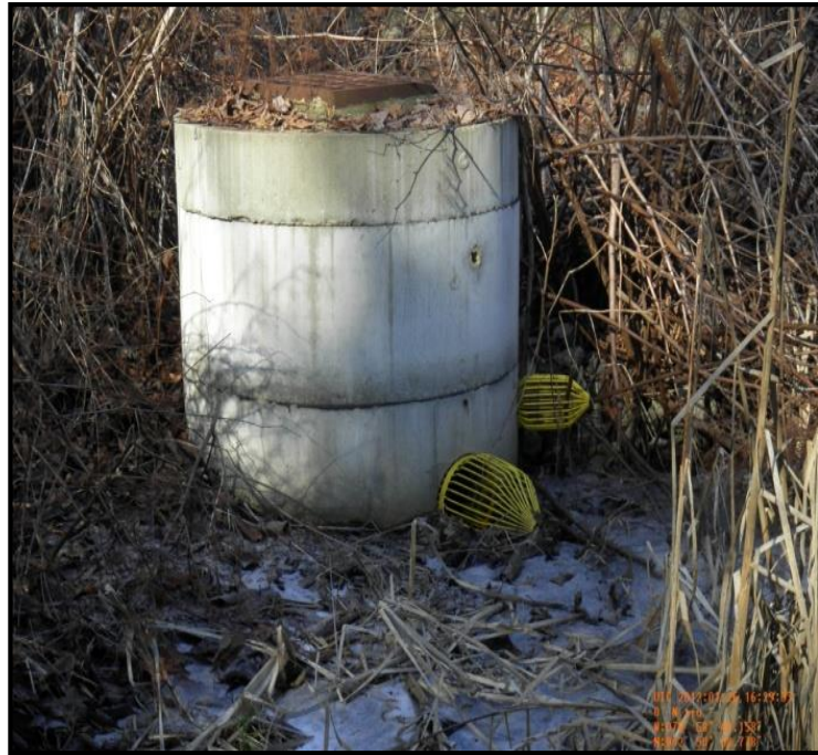
Figure 4-6: Sediment and debris filled in to level of yellow invert cages, short circuiting the detention BMP
