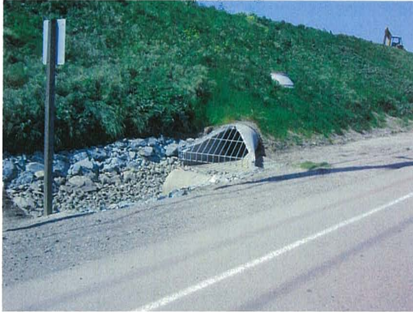
Photograph 5: Pacific Ethanol storm drain outfall into the drainage channel along Navy Drive.
