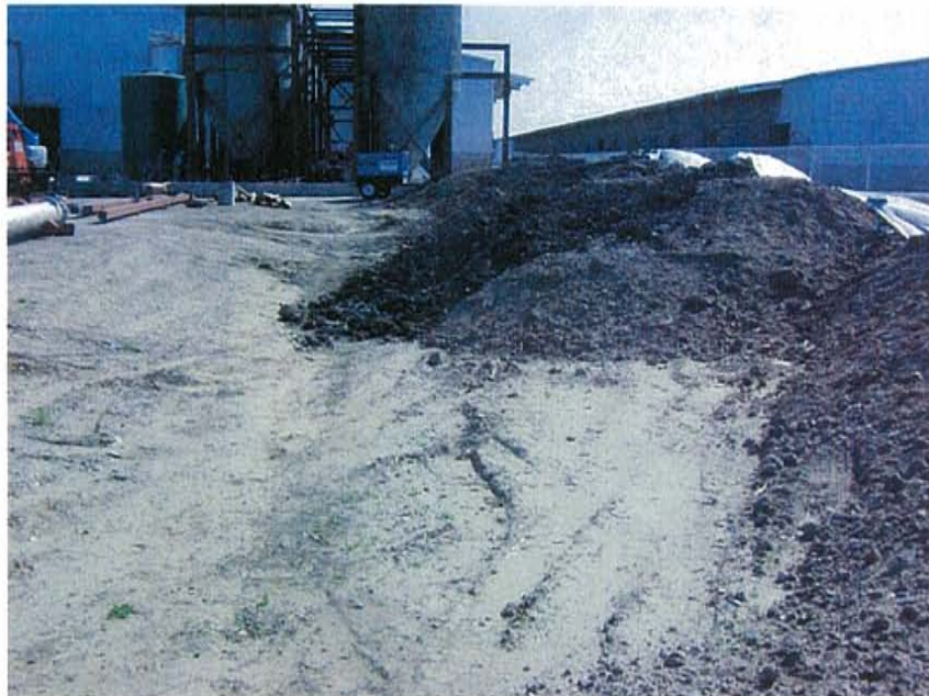
Photograph 10: In a follow-up audit activity on March 20, 2008, soil stockpiles were still located in a drainage pathway and temporary perimeter controls had not been installed.
