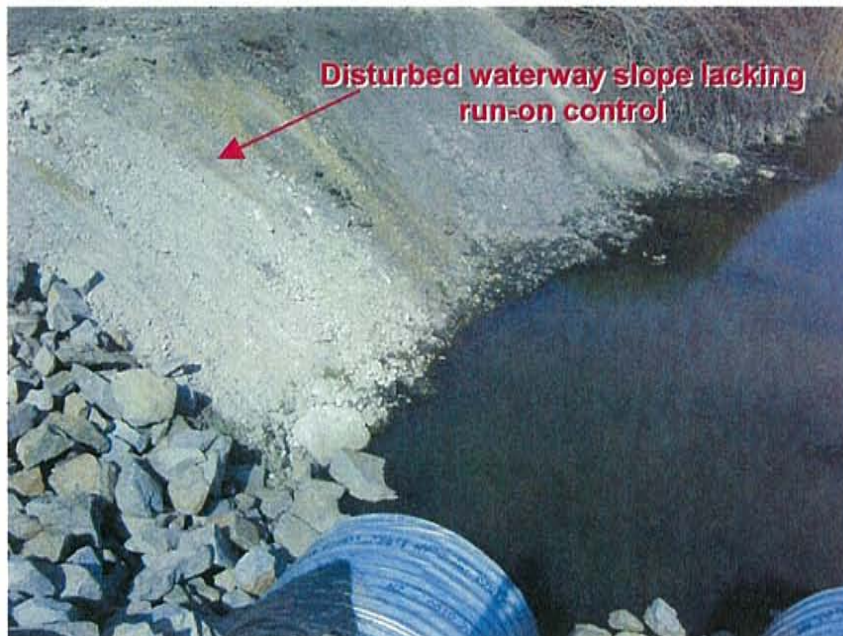
Photograph 8: Run-on control BMPs were not implemented between the disturbed area on the southwest side of the railway crossing and the adjacent unnamed waterway.
