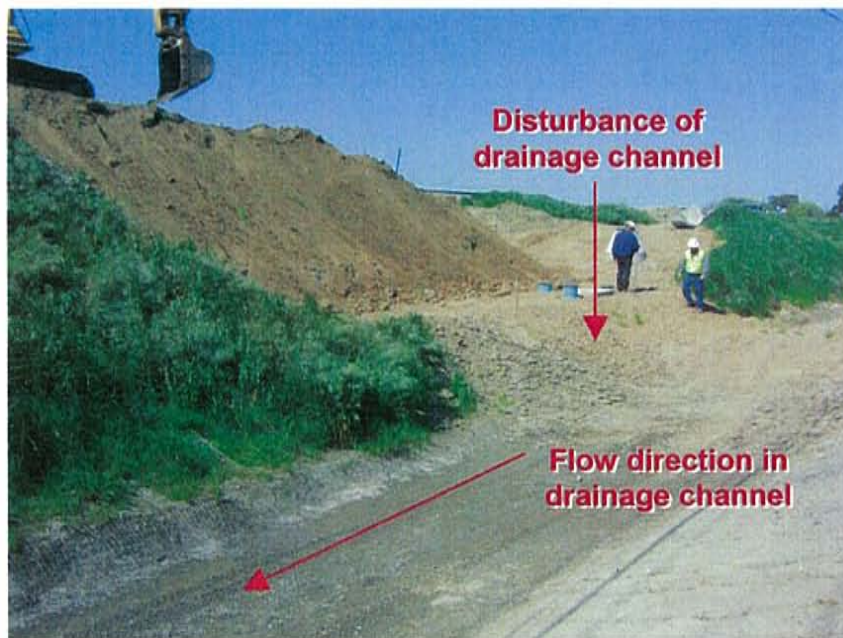
Photograph 2: BMPs were not implemented between the slope and the adjacent drainage channel or in the disturbed drainage channel itself, and the surface of the slope was not stabilized.
