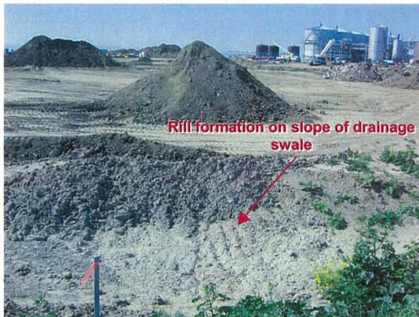
Photograph 4: Evidence of erosion was observed; including rill formation on the slope of the drainage swale.
