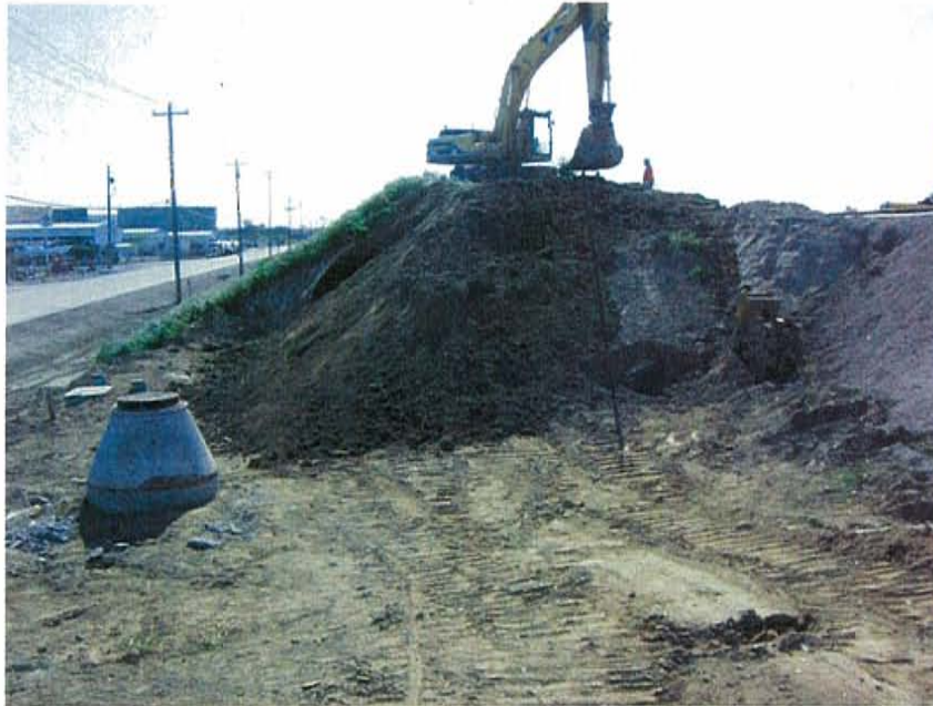
Photograph 1: An actively disturbed slope located adjacent to a drainage ditch along Navy Drive and southeast of the construction site entrance.
