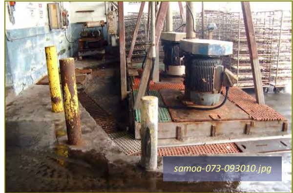
Photo #2: Dockside Central Pits - Pumps To WWTP Taken By: Greg V. Arthur Date: 09/30/10
