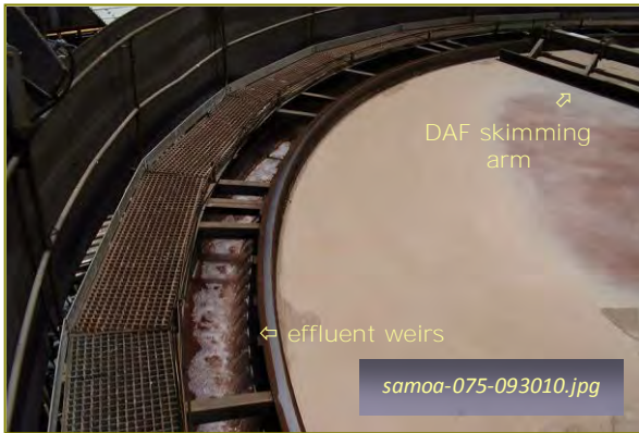
Photo #3: Dissolved Air Flotation Unit - Surface Weirs Taken By: Greg V. Arthur Date: 09/30/10
