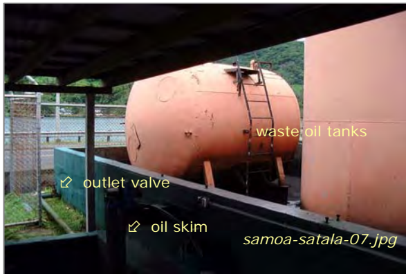
Photo #3: NPDES Sump #1 – Waste Oil Tanks Taken By: Greg V. Arthur Date: 04/01/08
