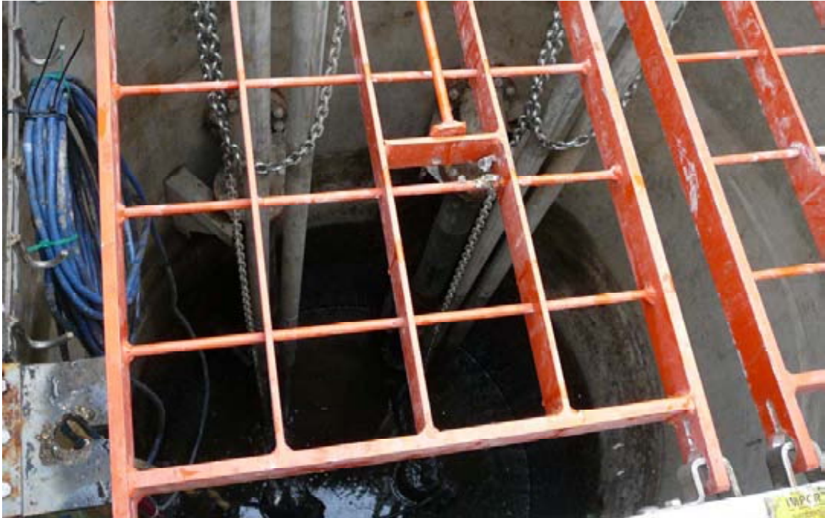
Berkeley Photo 1: Pump Station 7 wet well with safety grate.
