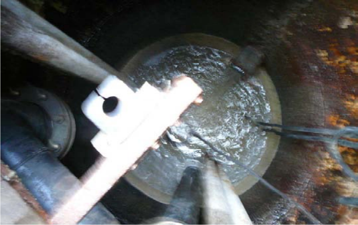
Berkeley Photo 5: Pump station 3 wet well.
