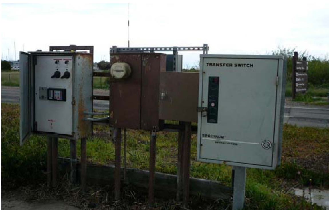
Berkeley Photo 4: Pump station 5 controls.
