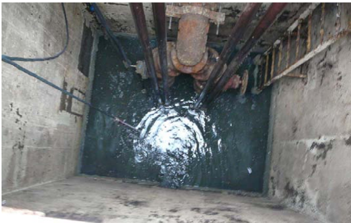
Berkeley Photo 3: Pump station 5 wet well.
