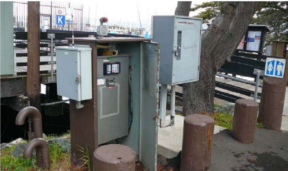
Berkeley Photo 6: Pump station 3 controls and transfer switch next to marina.
