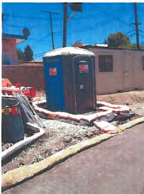
Photograph 10. Many Mansions Site Visit – View of portable toilet on visquine and lined with sand bags.
