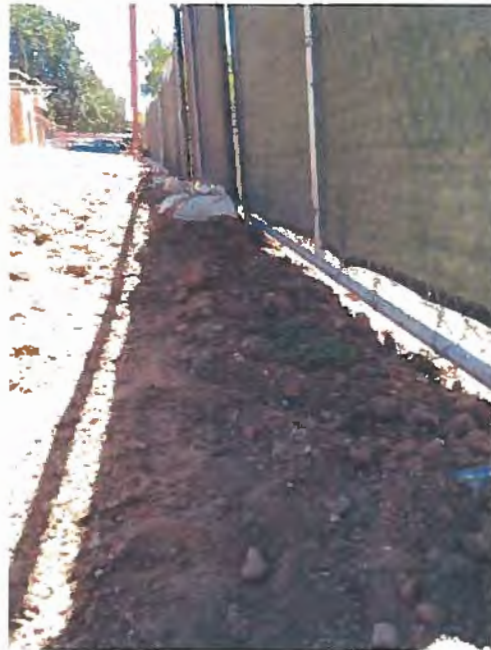
Photograph 7. Many Mansions Site Visit – View of soil on top of a retaining wall without sediment control BMPs to prevent soil from overtopping the retaining wall.
