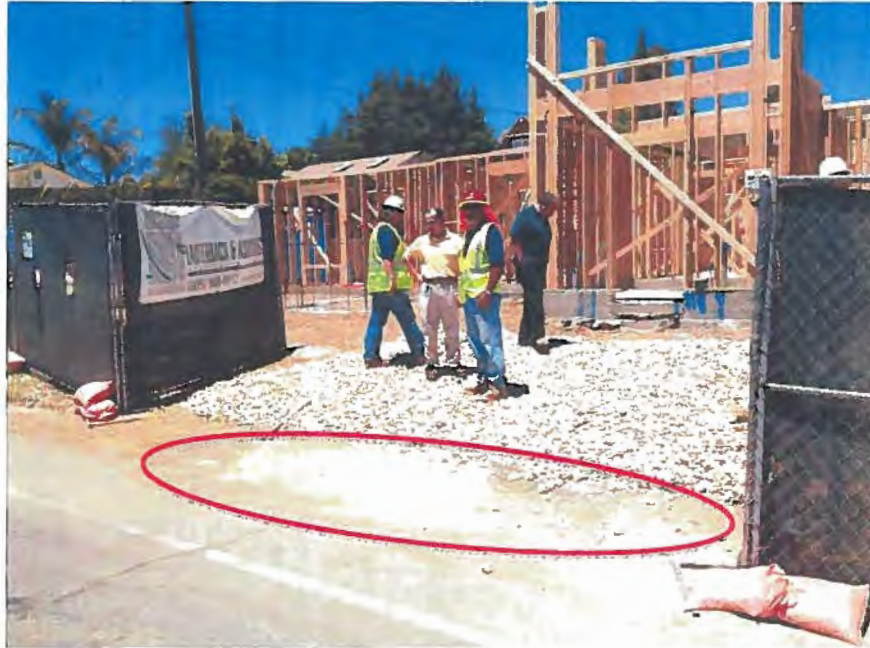
Photograph 3. Many Mansions Site Visit – View facing north on Los Feliz Drive of unstabilized soil outside the gate to the construction site.
