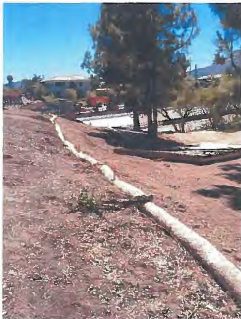
Photograph 5. Wendy Drive/101 Interchange Site Visit – View of fiber rolls installed along the slope of the embankment on the north side of Wendy Drive.
