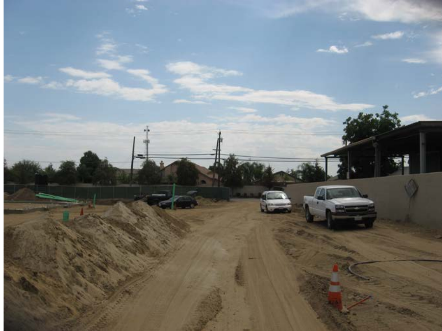
Photograph 1. View of southwest corner of the construction site. Note that the site had been initially graded and a contractor was installing building foundation pads at the time of the site visit.
