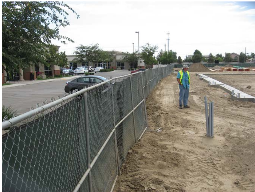
Photograph 2. View of the eastern perimeter of the construction site. Note that there is no silt fence to prevent sediment from leaving the site.
