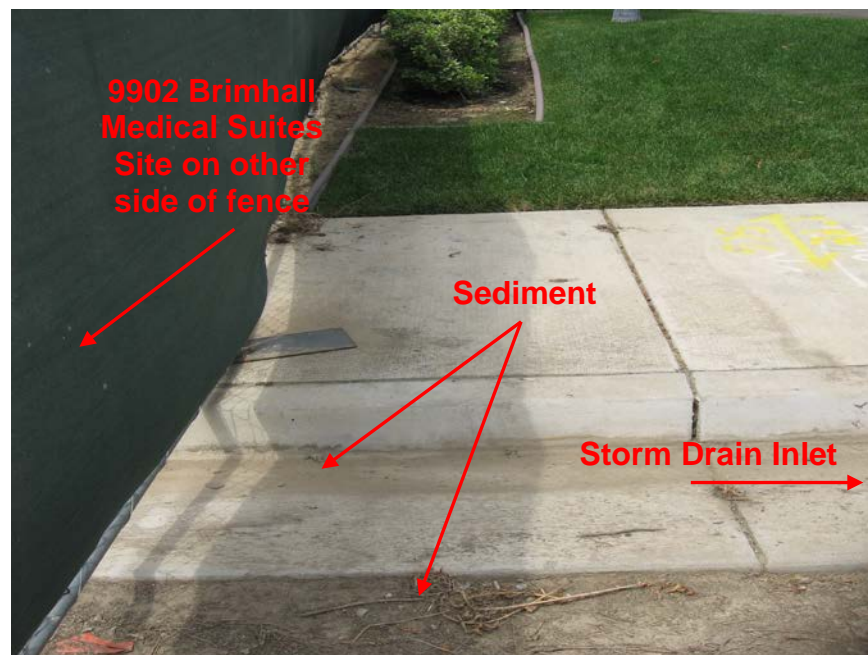
Photograph 4. Alternate view of sediment in curb and gutter flow line upgradient of unprotected storm drain inlet shown in Photograph 3. It was not clear to the EPA Inspection Team whether the drain inlet discharged to the City's MS4 or to a retention basin.
