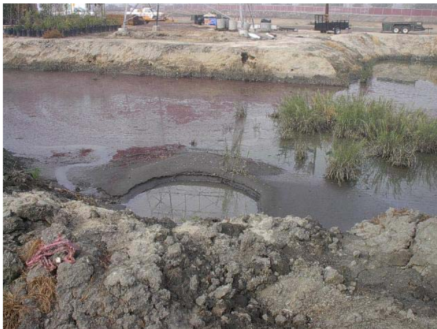
Photo 7: Detention pond in southern corner of yard. Pond is filled with sediment and other debris within about 3-4 feet of the top of the embankment. The pond was apparently recently excavated to remove some of the sediment and debris, which was placed on the embankment (bottom of photo).
