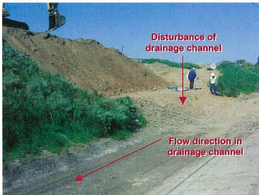
Photograph 2: BMPs were not implemented between the slope and the adjacent drainage channel or in the disturbed drainage channel itself, and the surface of the slope was not stabilized.
