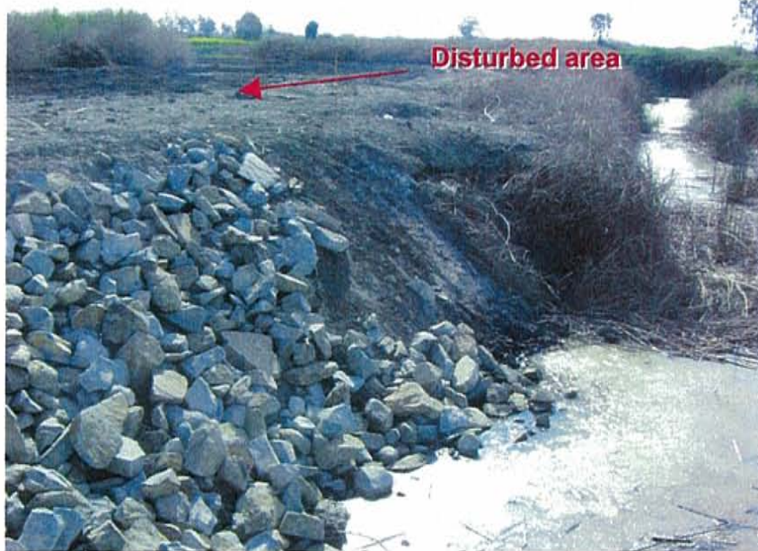
Photograph 7: BMPs were not implemented between the disturbed area on the northeast side of the railway crossing and the adjacent unnamed waterway.
