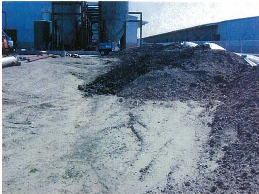
Photograph 10: In a follow-up audit activity on March 20, 2008, soil stockpiles were still located in a drainage pathway and temporary perimeter controls had not been installed.
