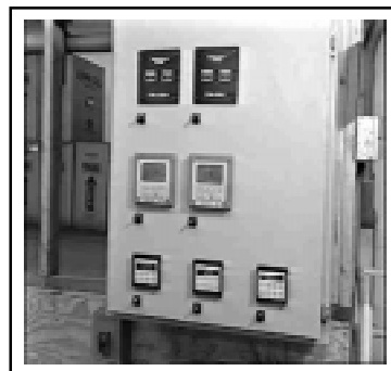
Figure 6. Analyzer Panel at the Artistic Facility
