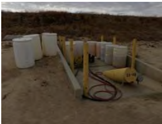
Olympus Stylus 8000, Photo #87; View of the leachate collection system and less-than-90-day storage area at WMU 33, Cell #4.
