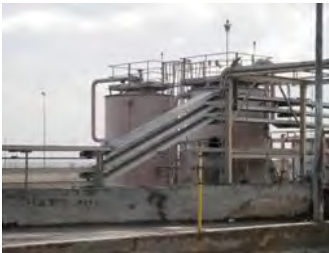
Olympus Stylus 8000, Photo #6; View of the RCRA-permitted water (left) and dirty water (right) storage tanks, facing southeast.
