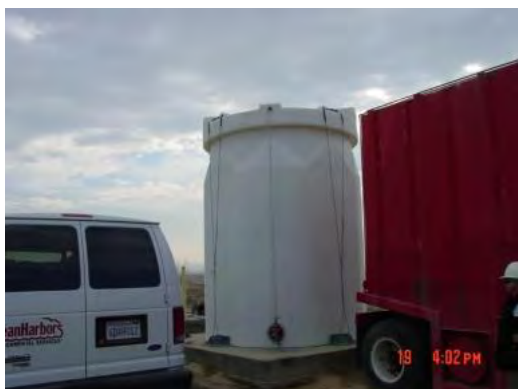
Sony DSC-S75, Photo #11; View of a 5,000-gallon, plastic, leachate collection tank at WMU 35, Cell #3, facing west.
