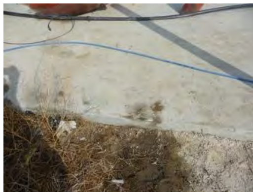
Panasonic Lumix DMC-TZ5, Photo #28; WMU 34; F039 leachate dripping on the ground.
