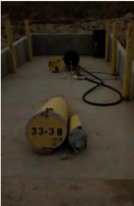
Olympus Stylus 8000, Photo #81; View of the leachate collection system at WMU 33 Cell #3B.
