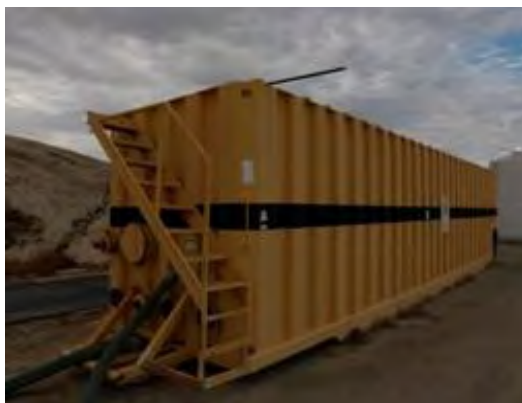
Olympus stylus 8000, Photo #96; leachate collection frac tank (Tank 80) at WMU 35 Cell #1.
