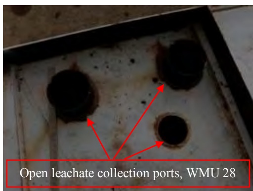
Olympus Stylus 8000, Photo #74; View of top of the leachate collection frac tank (Frac Tank 3) at WMU 28. Note the open ports.
