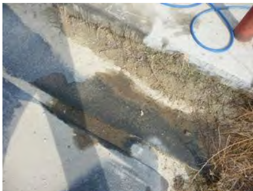
Panasonic Lumix DMC-TZ5, Photo #19; F039 leachate drippage observed on the ground at WMU 34.
