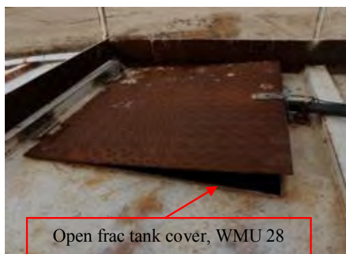
Olympus Stylus 8000, Photo #75; View of top of the leachate collection frac tank (Frac Tank 3) at WMU 28. Note the open cover.
