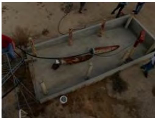
Olympus Stylus 8000, Photo #76; View of the leachate collection system at WMU 28 from the top of the leachate collection frac tank (Frac Tank 3).
