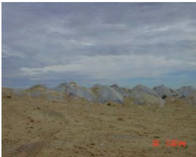
Sony Digital DSC-S75, Photo #13; View of the treated waste staging piles atop WMU 34 (under plastic tarping). View is from the southwest corner of WMU 34, facing east.
