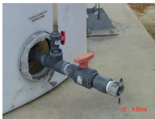
Sony DSC-S75, Photo #12; View of the piping and valve for draining the 5,000-gallon, plastic, leachate collection tank at WMU 35, Cell #3, facing northwest. Note: no secondary containment or cap/plug.
