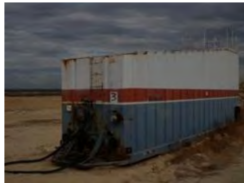
Olympus Stylus 8000, Photo #73; View of the leachate collection frac tank (Frac Tank 3) at WMU 28.
