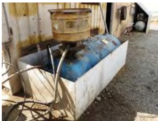
Olympus Stylus 8000, Photo #50; View of the used oil storage tank at the maintenance building.
