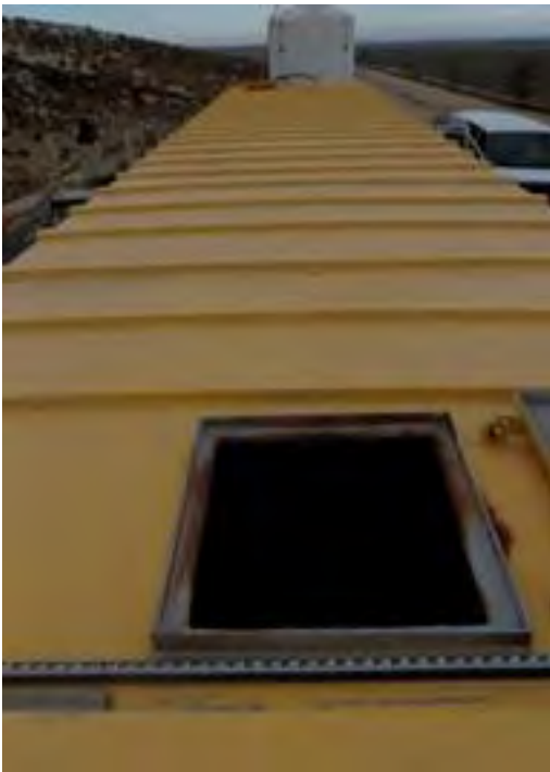
Olympus Stylus 8000, Photo #97; View of the leachate collection frac tank (Tank 80) at WMU 35, Cell #1. Note the top of the container is open.
