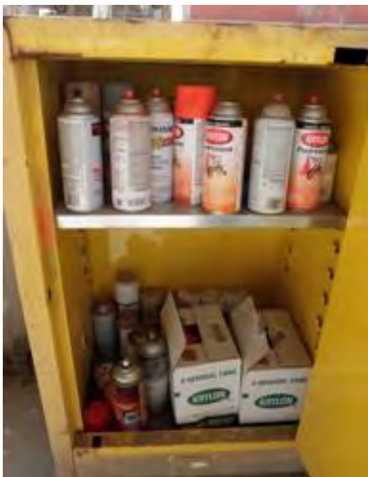
Olympus Stylus 8000, Photo #47; View of a flammable storage cabinet at the STU, holding aerosol products.
