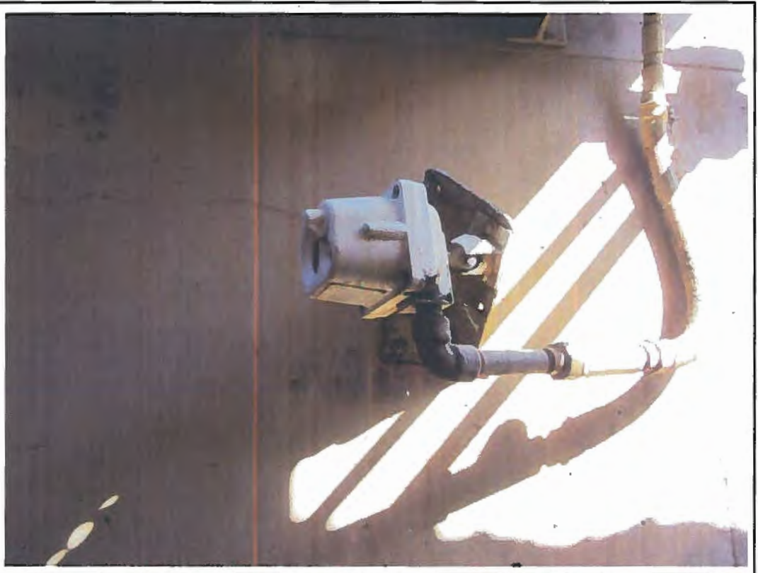
Photographer: CAIN Photo No. 5 Photo Description: Fire-Eye flame detector mounted in east end of well gallery
