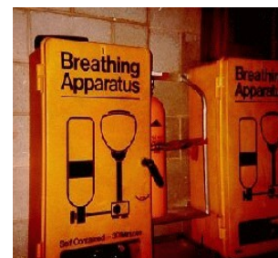
Inspect Emergency Equipment Regularly
