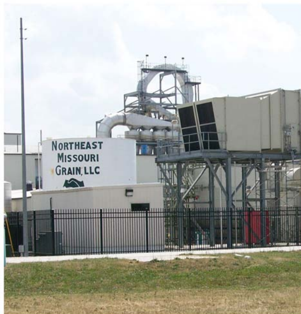
Award-winning cogeneration plant in Missouri
