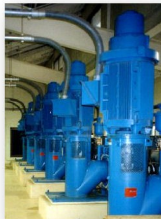
Drinking Water Intake Wells
