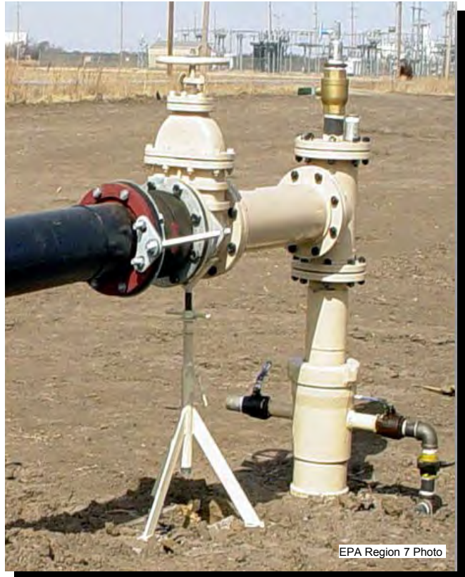
UNDERGROUND INJECTION CONTROL WELL HEAD
