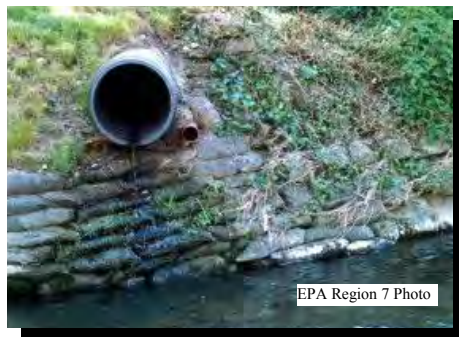
DIRECT DISCHARGE OF WASTE INTO A SURFACE WATER BODY CONTRIBUTES TO WATER POLLUTION
