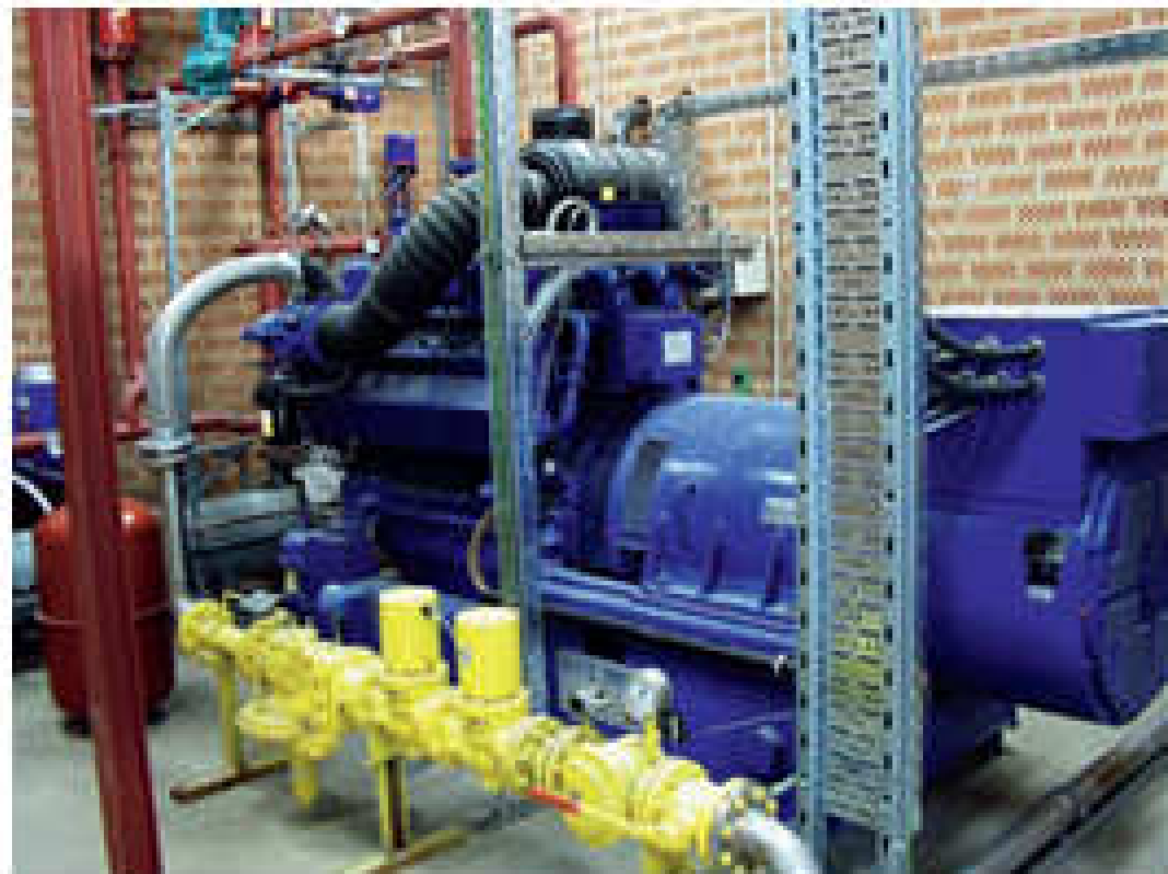
Example CHP unit inside building
