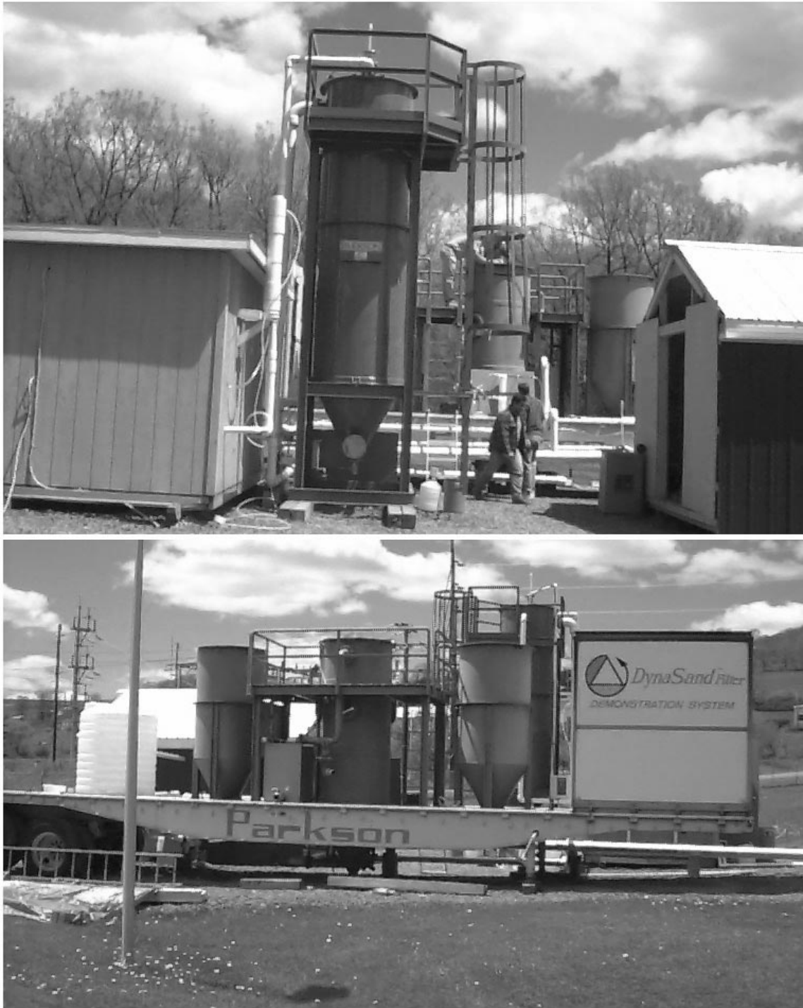
Figure 3.7 CBUD sand filtration facility.
