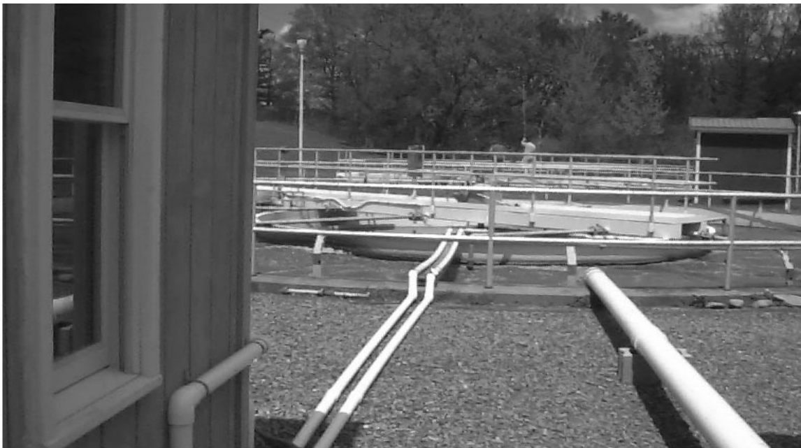
Figure 3.3 Demonstration influent drawn from secondary clarifier.
