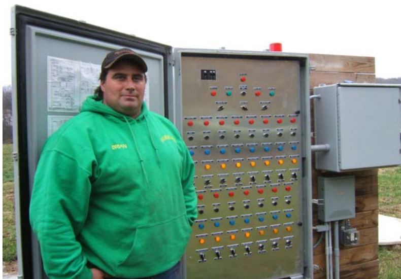
Figure 1.13 Brian McIntosh, operator of the new Bovina Community Septic System, at the control panel, where flow from the settling tanks is directed to twelve leach fields. Photo courtesy of Catskill Watershed Corporation
